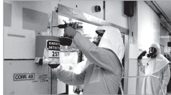
Workers prepare to remove four gloveboxes from PFP. Funding from the American Recovery and Reinvestment Act will help DOE complete demolition of PFP by 2013, three years ahead of schedule.
