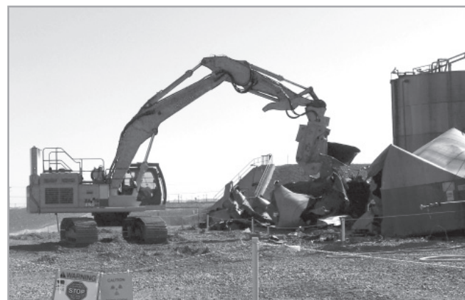
Crews demolish large tanks near U Plant on the Central Plateau. This work is funded by the American Recovery and Reinvestment Act.
