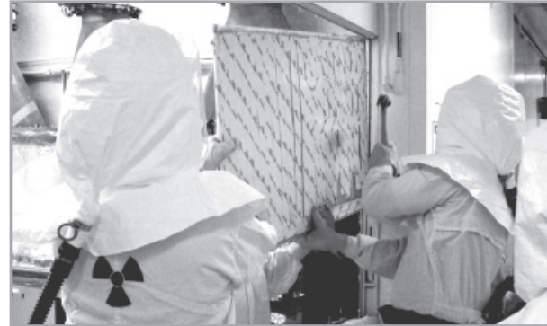
Workers remove a section of the wall at the Plutonium Finishing Plant. Hanford recently celebrated moving all plutonium and reactor fuel containing plutonium out of PFP.
