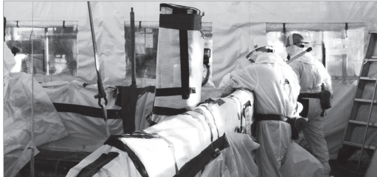
Workers completed construction of the waste retrieval system for tank C-104 at Hanford in 2009.
