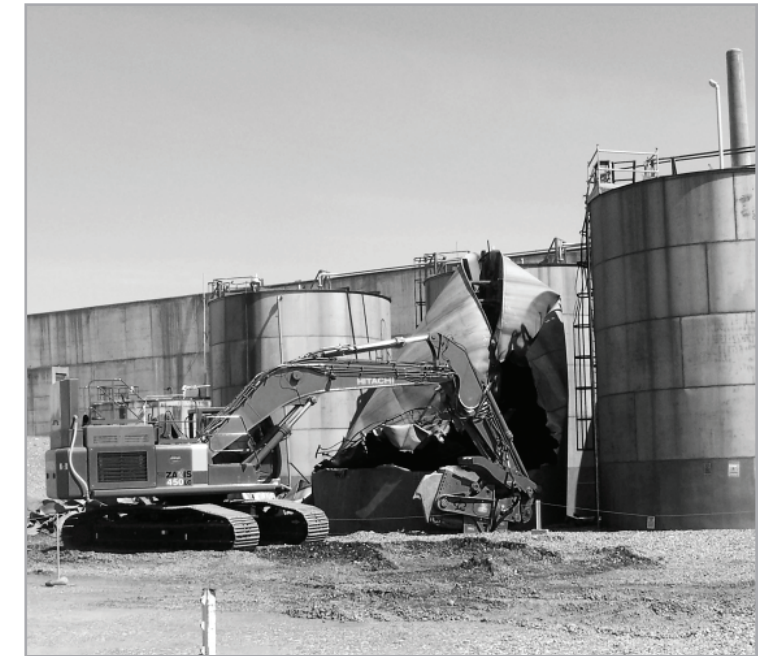
Crews demolish large vertical tanks at N Area. This work is part of the effort to shrink the active cleanup footprint of the Central Plateau.
