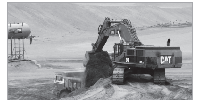
An excavator removes stockpile dirt from an area where new disposal cells will be developed at ERDF, the disposal facility for mixed low-level waste. This work is funded by the American Recovery and Reinvestment Act.
