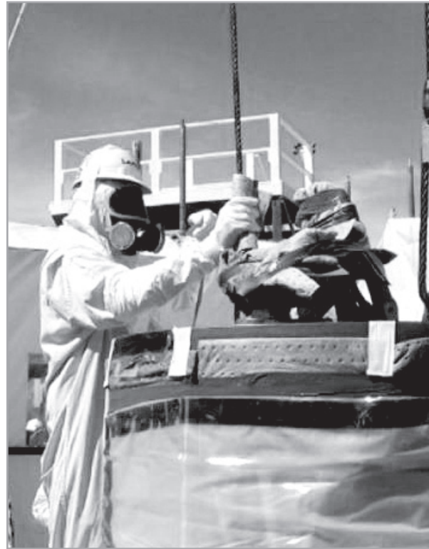
Construction was completed on the waste retrieval system for tank C-104 at Hanford. The proposed settlement agreement between the TPA agencies would change the deadline for retrieving all waste from C Farm single-shell tanks to 2014 instead of 2006.
