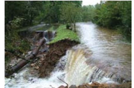
Damage to the city water system in Asheville, North Carolina, due to heavy rain in 2004.
