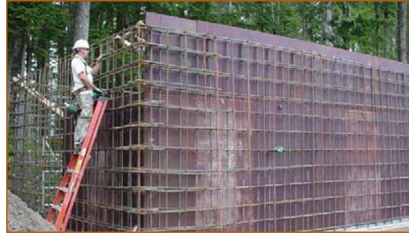
Figure 15: Sedimentation tank rebar and forms. An estimated 80,000 pounds of rebar was required for the construction of the sedimentation tank and building.
