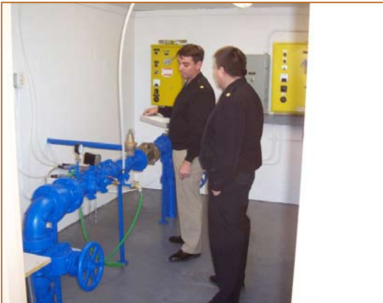
Figure 4: IHS engineers at the final inspection for pumphouse expansion for Desmet community, ID.
