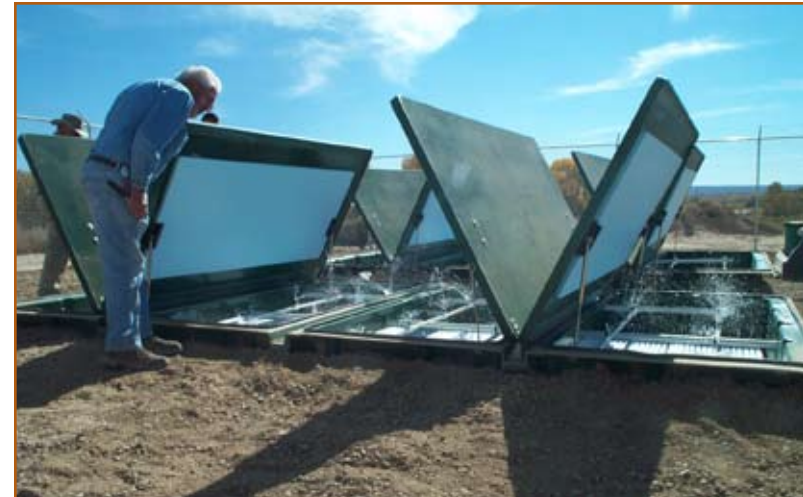
Figure 8: Startup of an Advantex water reclamation facility serving 20 homes, NM.
