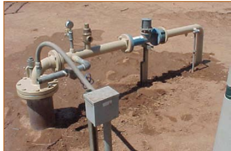
Figure 28: Upgraded well pumps and piping.
