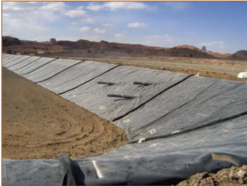
Figure 7: Wastewater treatment lagoon in Kayenta, AZ.
