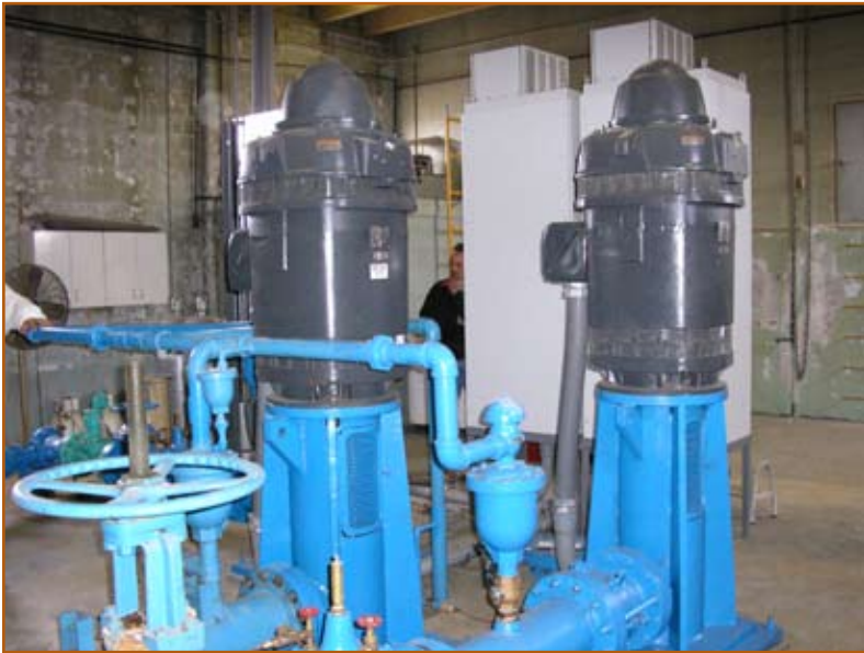
Figure 42: Pair of 200 hp pumps at the Fox Ridge WTP.
