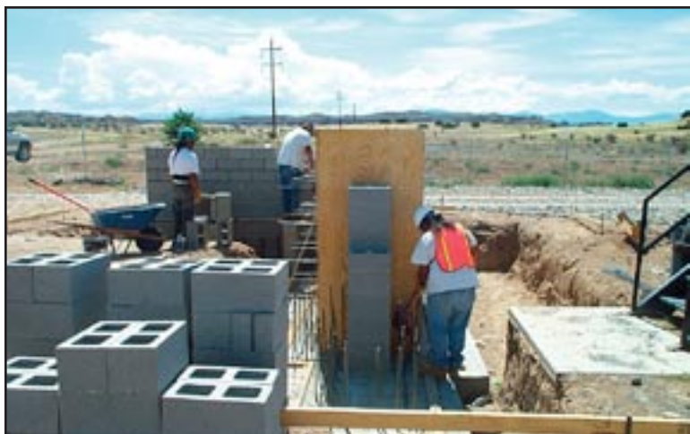
Figure 47: Construction of a new headworks and grit removal system at the San Juan Pueblo, New Mexico.
