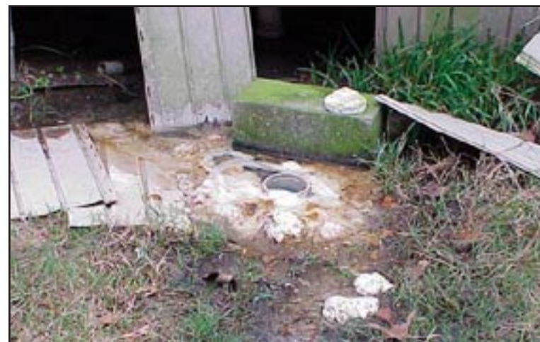
Figure 28: Example of surfacing sewage that has been eliminated by this project.
