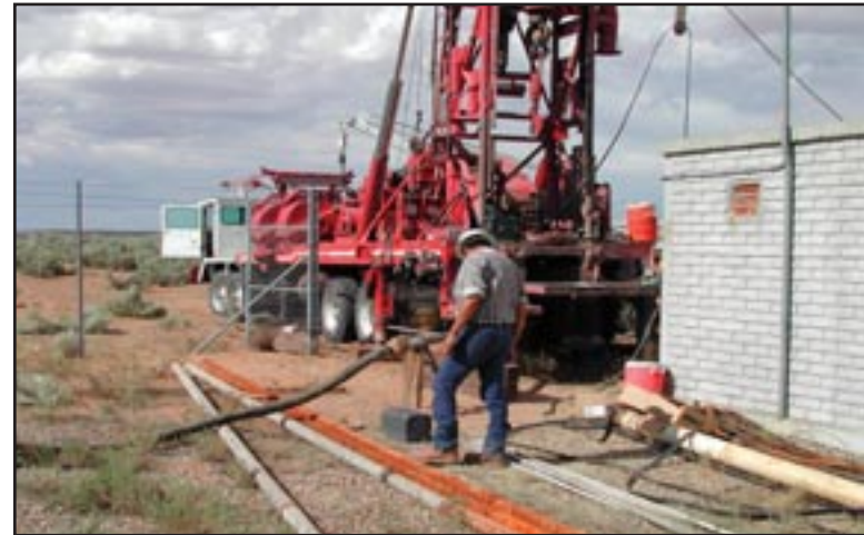
Figure 46: Chester Lapahie of the Farmington, New Mexico field office does test pumping at Ojo Encino on the Navajo Reservation, New Mexico.
