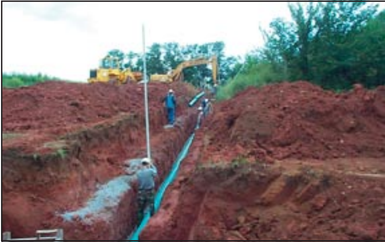
Figure 33: Checking sewer main grade to accurately tie into existing sewer by old lagoon.
