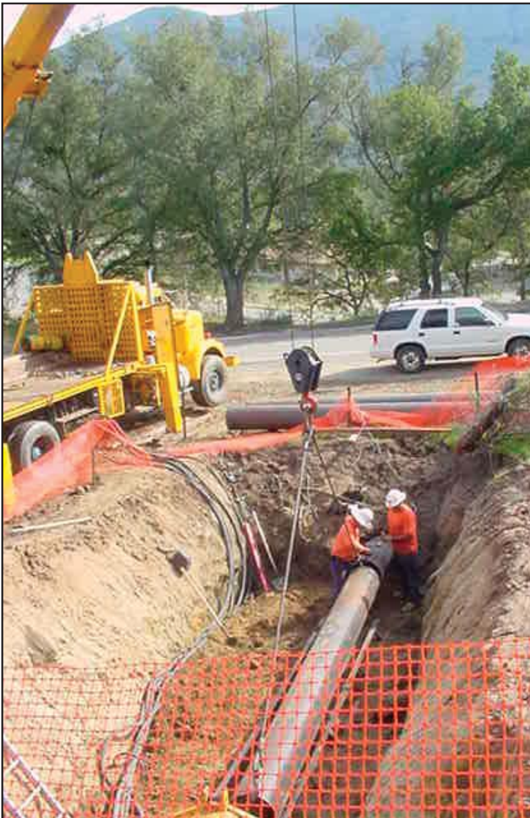
Figure 7: : Road bore as part of a 4 mile water main installation on the La Jolla Reservation, California.
