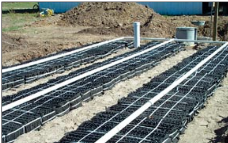
Figure 40: An Eljen in-drain leachfield system installed for a new homeowner in Taos Pueblo, New Mexico.
