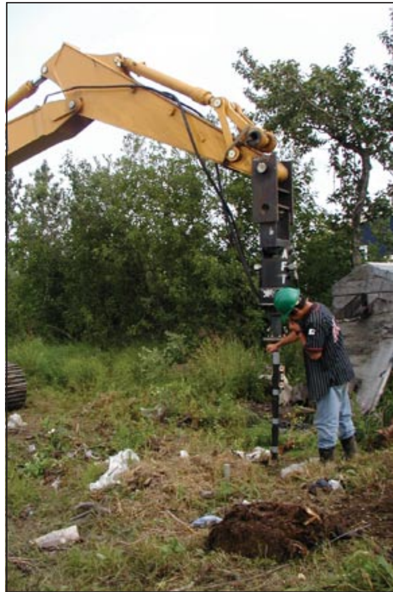
Figure 44: The Kwethluk crew installs helical anchors which will be the foundation for the above-ground utilidor, Alaska.
