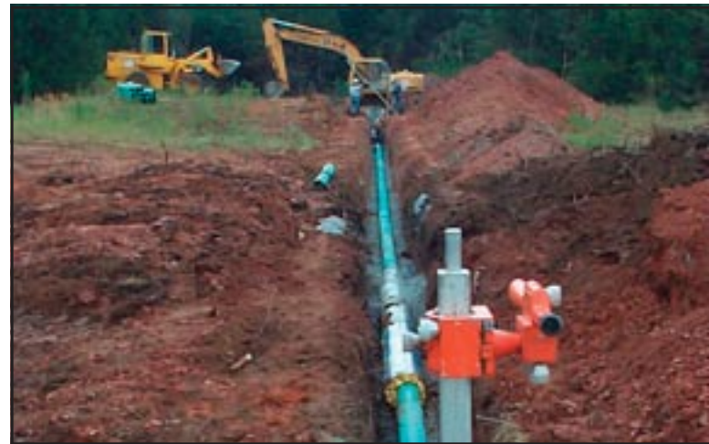
Figure 32: Construction of sewer main from junction manhole to daycare/elderly housing with insulated pipe.
