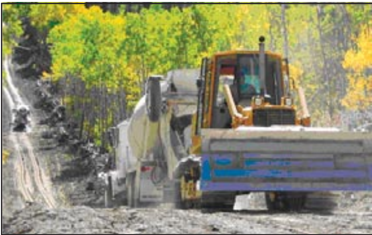
Figure 9: Bulldozer pulls a cement truck uphill while second truck waits at the bottom of the hill.
