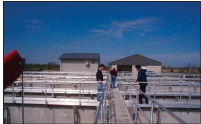
Figure 8: Startup of the mechanical wastewater treatment plant at Sac and Fox, Iowa.
