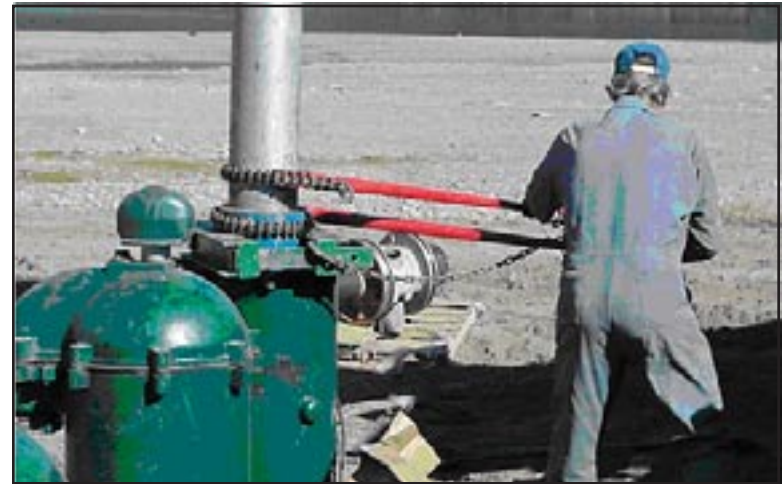
Figure 10: Intake pump fittings and pipe being assembled which the connections torqued to 3,500 ft-lb.
