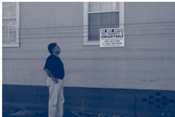
HUD Inspector General Kenneth Donohue stands below waterline viewing damage at Abundance Development.
