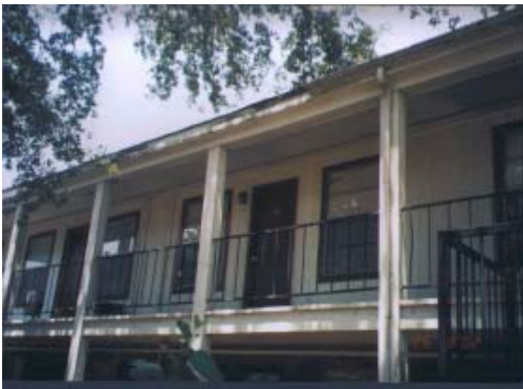
Missing gutter and rotted fascia boards at Colonial Oaks project.
