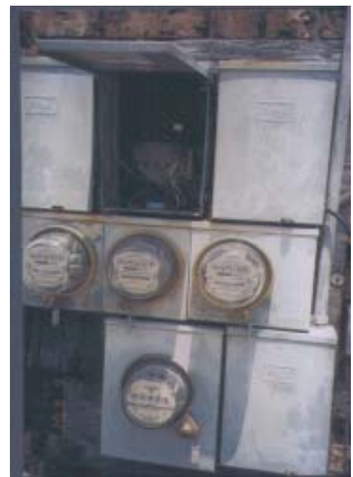
Missing breaker box cover and exposed wiring at Colonial Oaks project.
