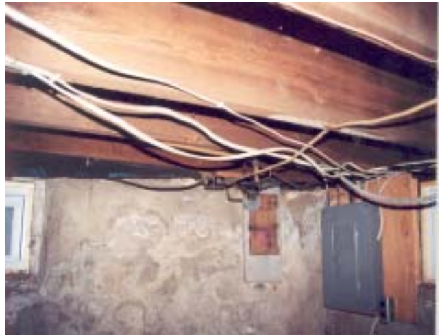
Example of housing rehabilitation work that was improperly performed at one of Housing Continuum's projects. Electrical wiring not installed in conduit.
