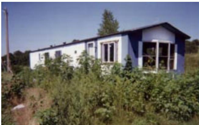
Mobile home purchased with Indian Housing Block Grant funds. Home was not inspected prior to purchase.
