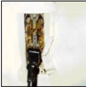
Missing cover plate caused exposed wires of electrical outlet.
