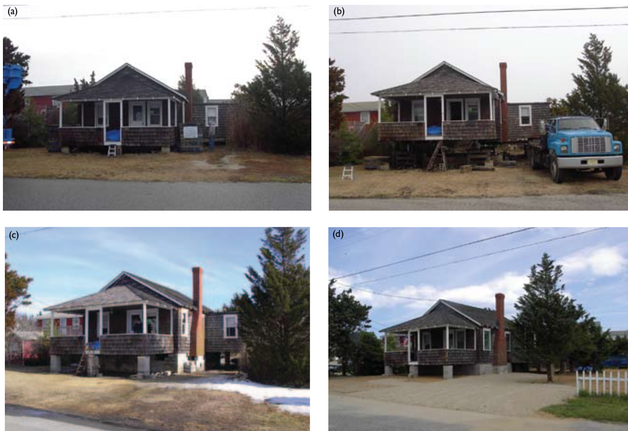
Figure 12.5 Elevating land and house (January through June 2005). (a) Initial elevation of house in Brant Beach, New Jersey. (b) Structural beams placed under house, which is lifted approximately 1.5 meters by hydraulic jack in blue truck. (c) Three course of cinder blocks added then house set down onto the blocks. (d) Soil and gravel brought in to elevate land surface. [Photo source: ©James G. Titus, used with permission].
