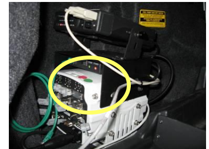
Installed Unit in Vehicle Trunk
