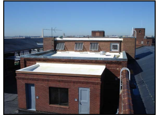
GPO used biobased roof coatings to help prolong the life of the roofs.
