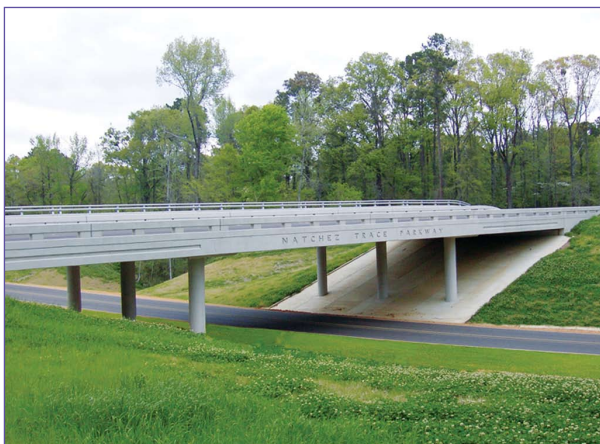
Natchez Trace Parkway over Palestine Road, Adams County, Mississippi (National Park Service)
