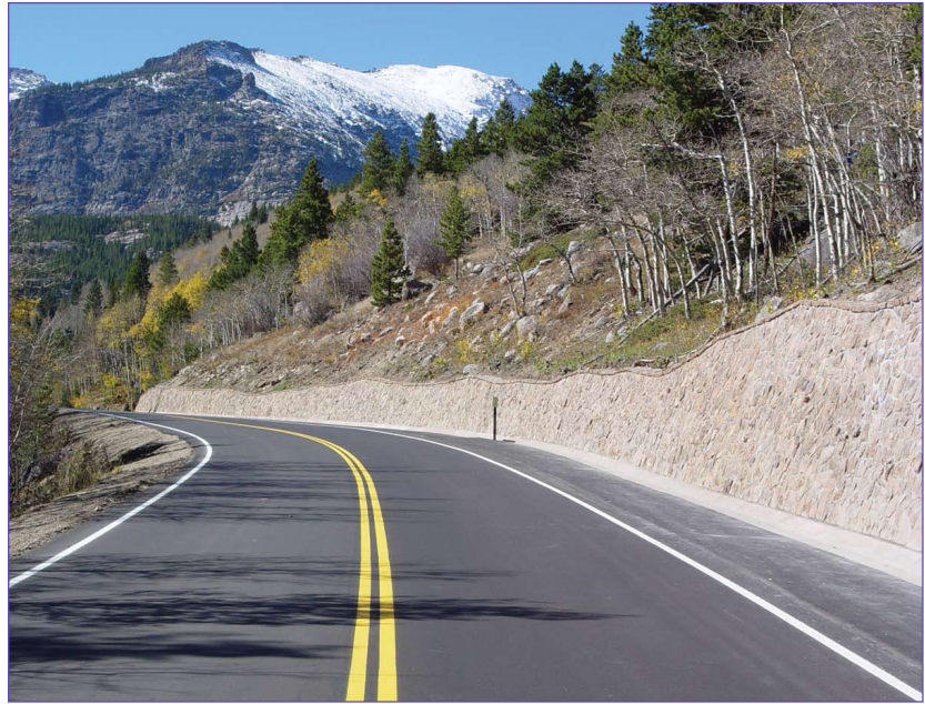
Use of real stone facing blends the retaining walls with the terrain. Bear Lake Road, Rocky Mountain National Park, Colorado (National Park Service)
