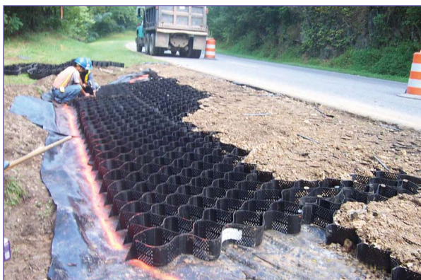
Placement of Geoweb—Green Parking Area Alternative, Great Smoky Mountains National Park, Tennessee (National Park Service)
