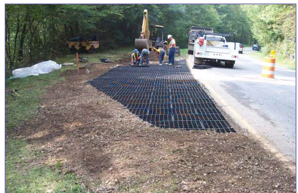
Placement of Geoblock—Green Parking Area Alternative, Great Smoky Mountains National Park, Tennessee (National Park Service)
