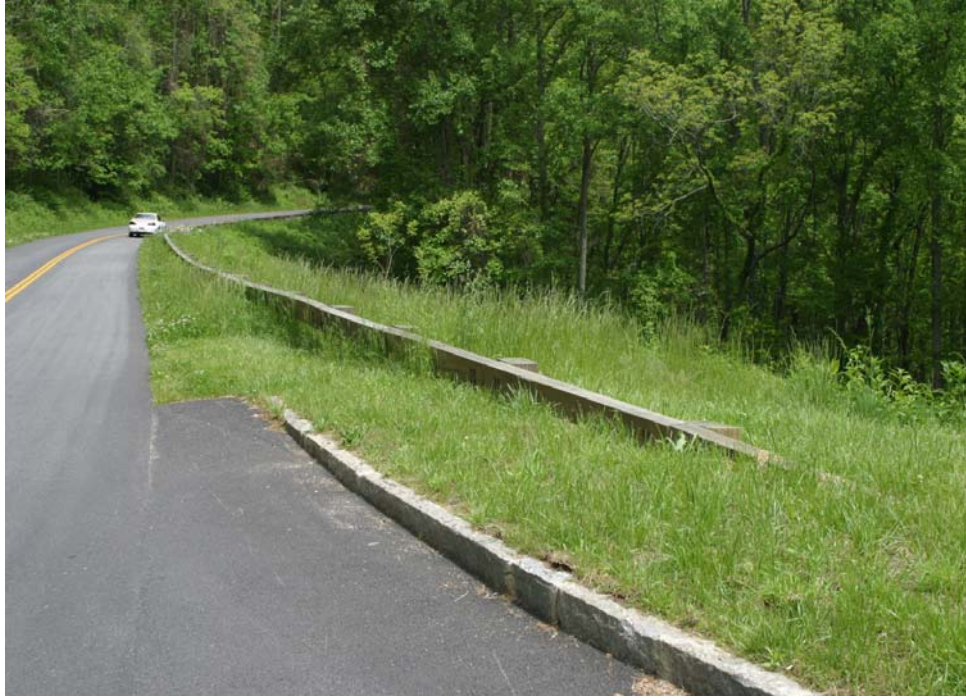
Timber guardrail standard height is not maintained up to the FAT-30 terminal section.
