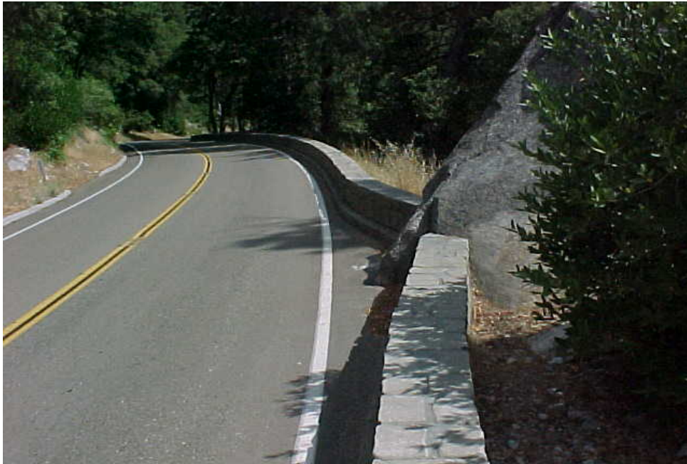
Rock protruding into the roadway. Guardwall ties into protruding rock. Typical problem of environmental challenges during project design and construction.
