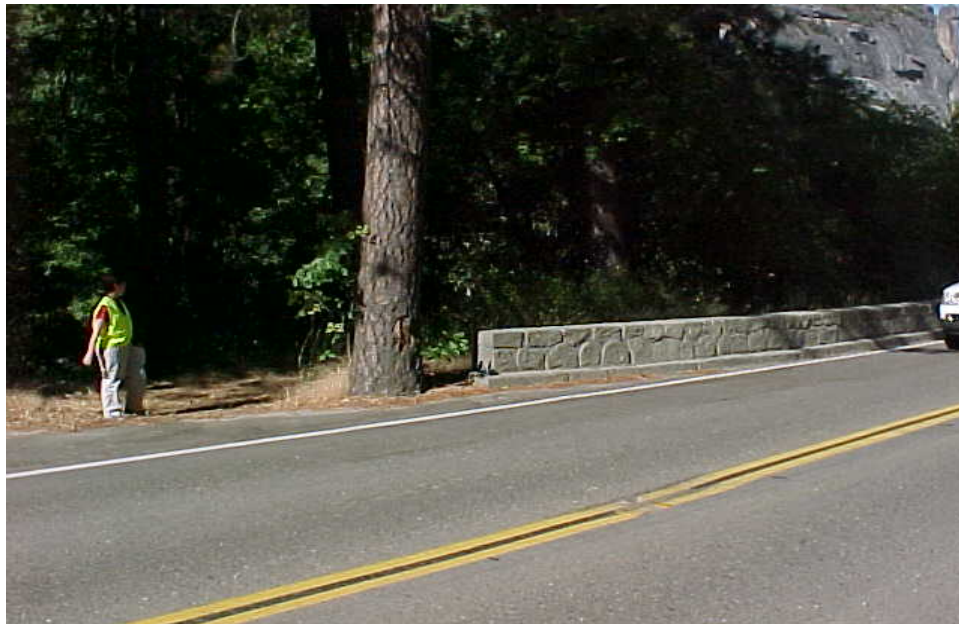
Guardwall terminating at a tree, within clear zone for opposing traffic.
