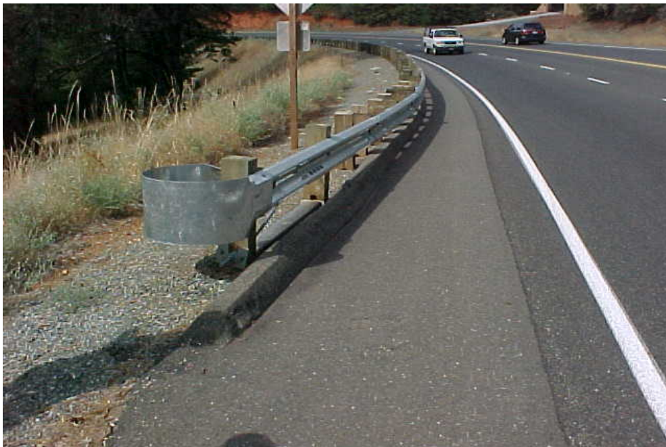
Curb in front of Slotted Rail Terminal (SRT) which negatively affects performance of the terminal section.
