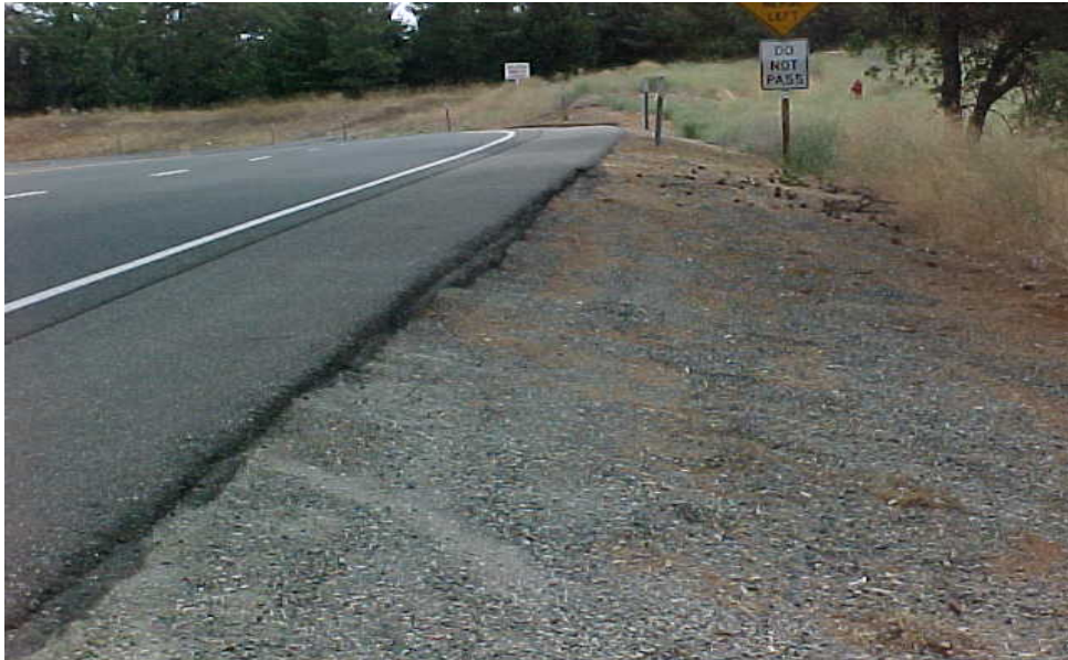
Example of improper signing as the warning sign is above a regulatory sign on the same Post. Also note the pavement drop-off is greater than 2 inches.
