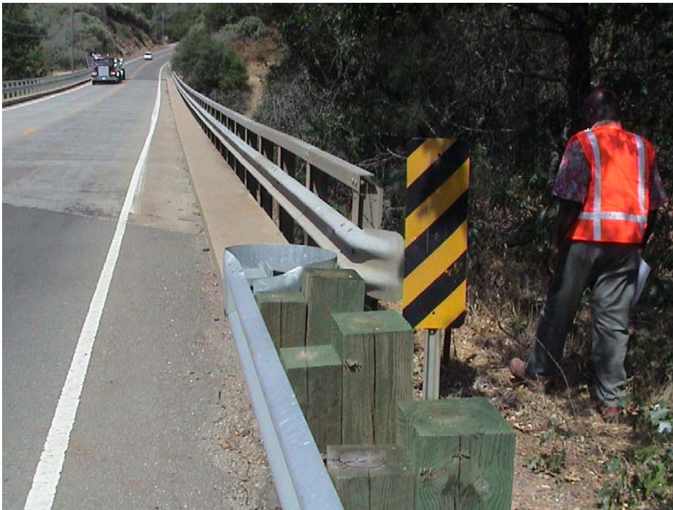
Guardrail approach transition to bridge railing is not crashworthy. Offset of guardrail in front of bridge is a potential hazard for opposing traffic.
