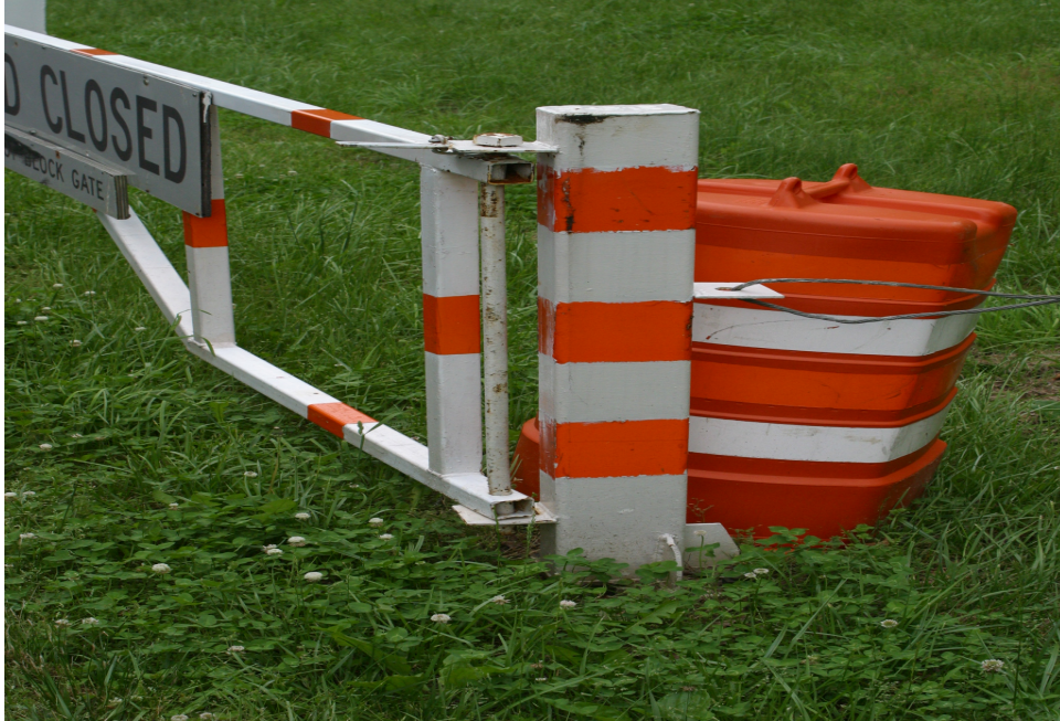
Entrance gate post within clear zone (approximately 2-feet from travel lane) is non-crashworthy
