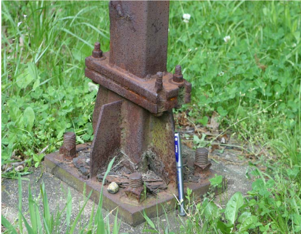
Severely rusted breakaway bond plate connection needs replacement. Also, the bond plate height is greater than 4-inches from the concrete footing.
