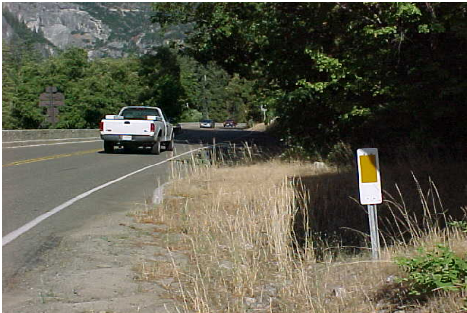
Incorrect placement of Object Marker. Object Marker about 3 meters off shoulder.
