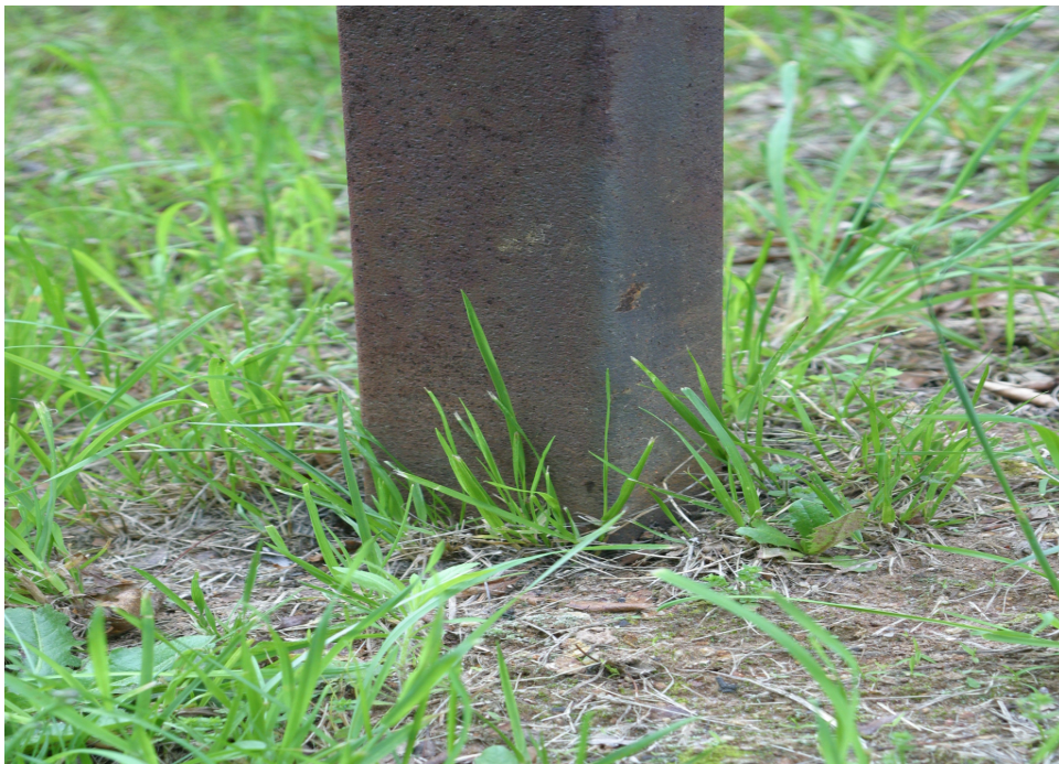
Weathering steel sign post installed without breakaway design.
