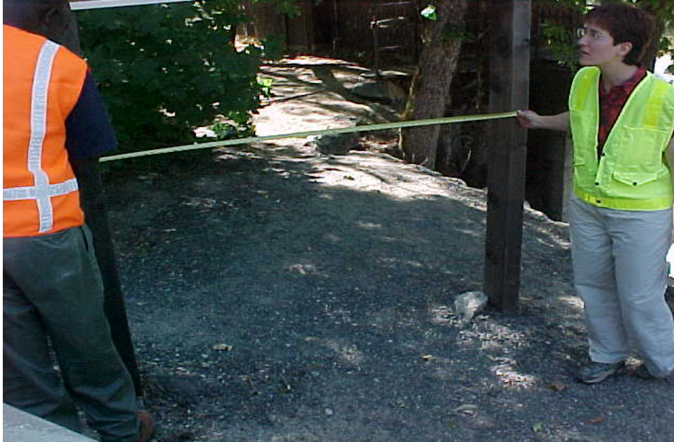
4" x 6" wood posts installed without breakaway holes in posts within the clear zone, and are not considered to be crashworthy.
