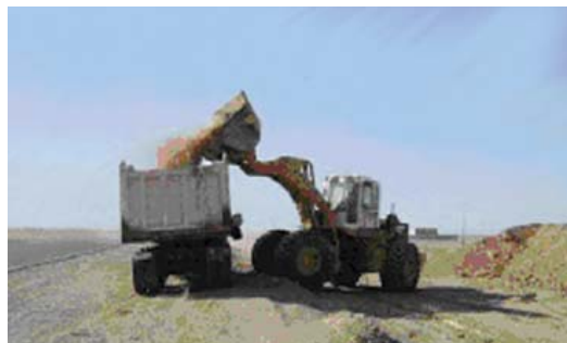
Work on the southern segment of the Baghdad-Kirkuk Carriageway was stopped when the project was 89% complete. (USACE photo)
