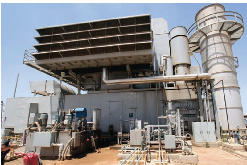
Site Photo 9. General Electric LM-6000 turbine unit.
