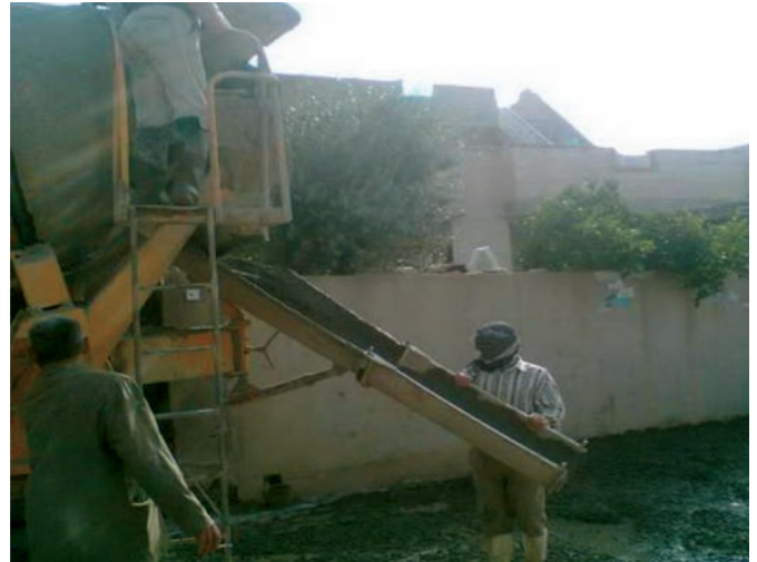
Site Photo 13. Aggregate base and concrete base pour (photo courtesy of USACE).
