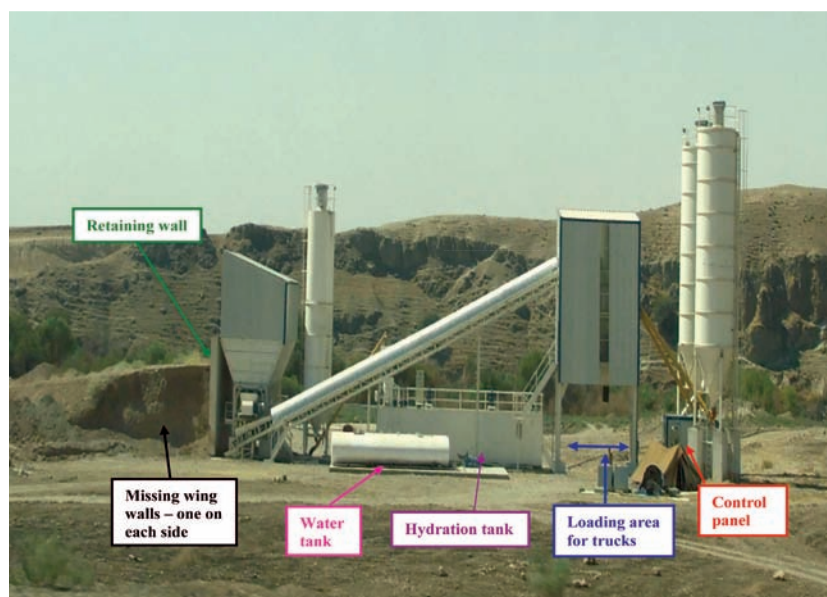
Site Photo 5. View of the “modified” 100-m 3 /hour grout-mixing plant.
