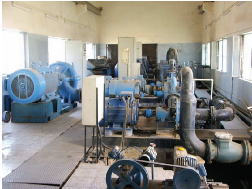
Site Photo 16. General maintenance on the interior of the booster pump room.
