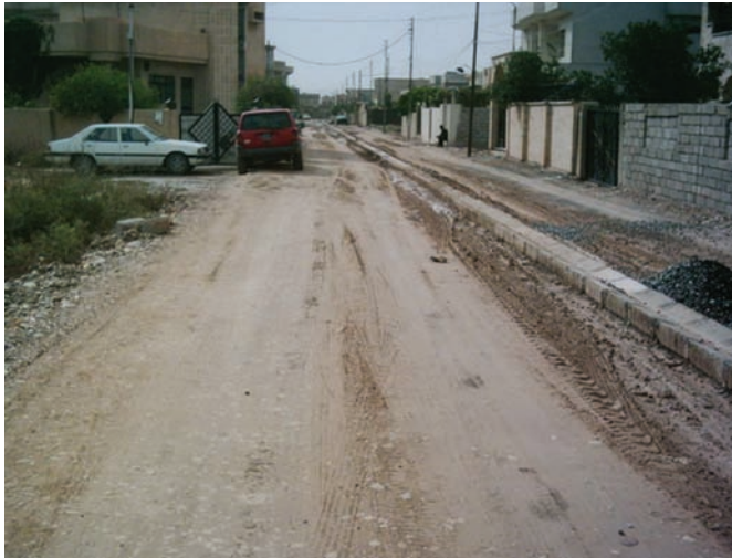
Site Photo 12. Road excavation, leveling, and rolling of the sub-grade (photo courtesy of USACE).
