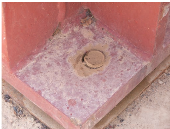
Site Photo 4. Close-up view of foundation bolts for the stationary silos.
