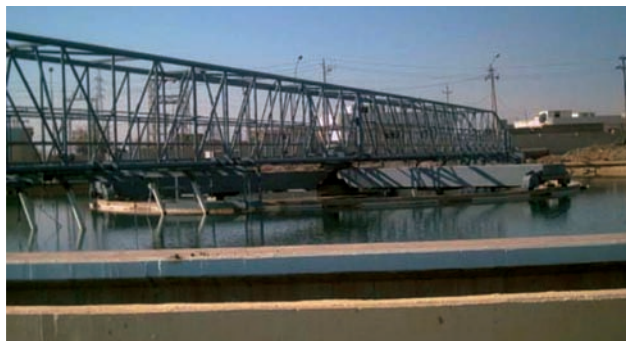
Site Photo 15. Settling tank (photo courtesy of USACE).
