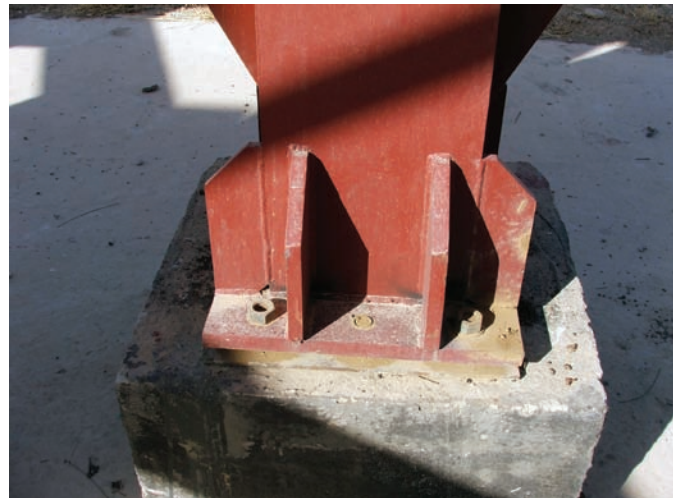
Site Photo 3. Close-up view of foundation bolts for the stationary silos.
