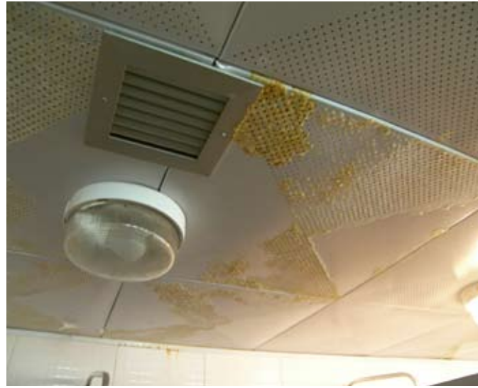
Site Photo 34. Crystallized urine on ceiling tile.
