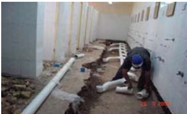
Site Photo 8. Extensive rework was required in dormitories to install watertight plumbing fittings. (Photo courtesy of ECCI)
