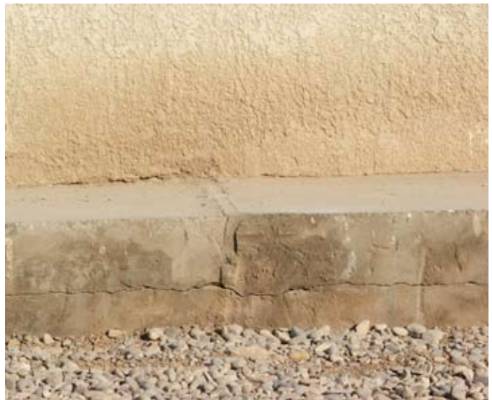
Site Photo 13. Close-up of the horizontal foundation fracture in the East Barracks.
