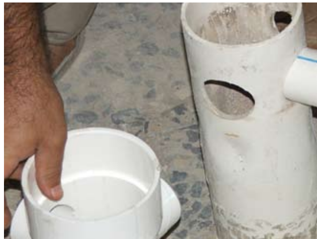
Site Photo 36. Contract-specified wastewater pipe connection is shown on the lower left.
