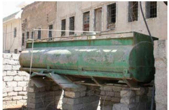
Site Photo 20. Old fuel truck tank placed by IP to supply the generator.
