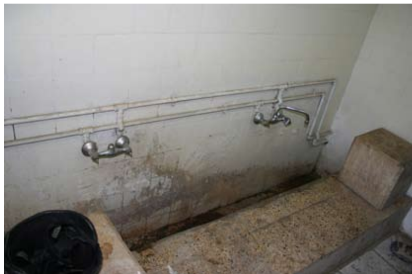
Site Photo 16. Existing wall tile was painted, and existing leaking faucets were not replaced. The left faucet in the photo's center was capped/disabled rather than replaced as required.
