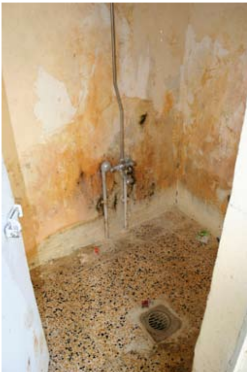
Site Photo 15. Painted plaster shower wall should have been grouted tile, floor to ceiling.
