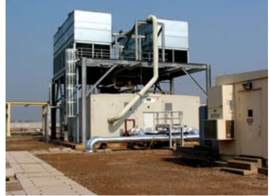
Al Qudas Power Plant
