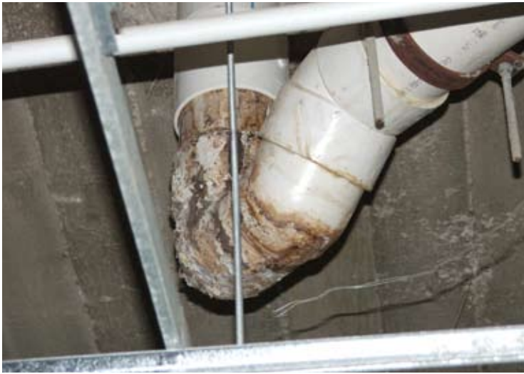
Site Photo 31. View of pipe leaking wastewater.
