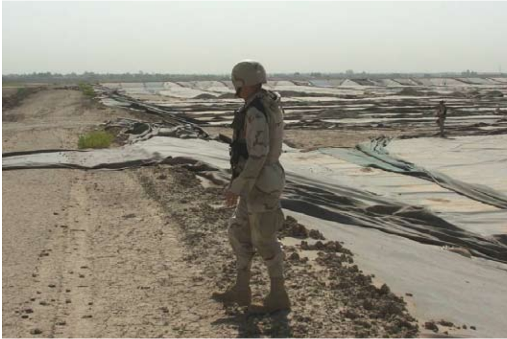
Site Photo 6. Section of the perimeter berm requiring remedial work to anchor the liner.
