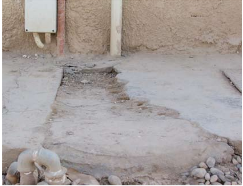
Site Photo 11. Substandard patchwork in Academy HQ sidewalk.
