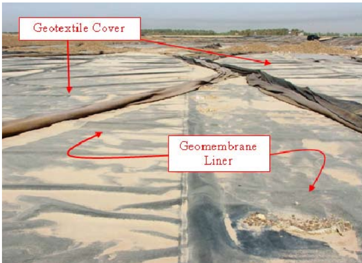
Site Photo 4. Exposed geomembrane liner.
