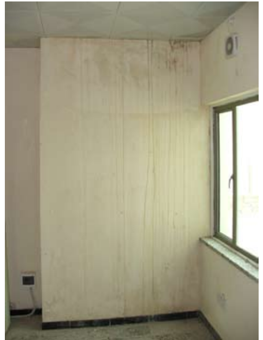
Site Photo 32. Damage to the wall from leaking wastewater.
