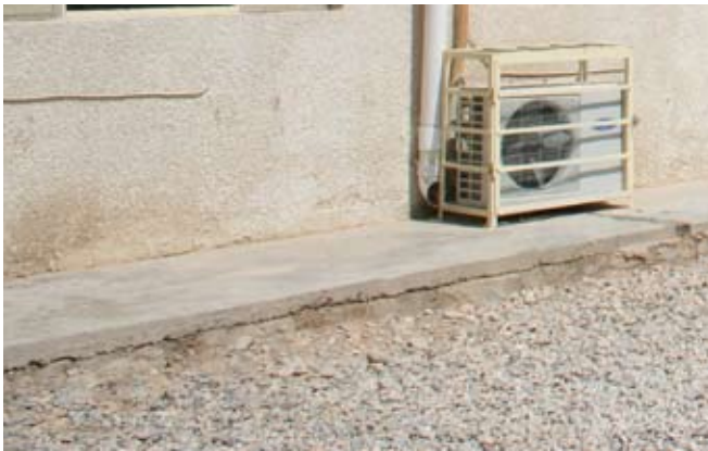
Site Photo 12. Horizontal fracturing along foundation of Middle Barracks.
