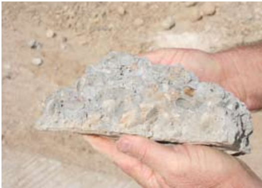
Site Photo 10. Weak and crumbly concrete piece pulled from roadway by hand.
