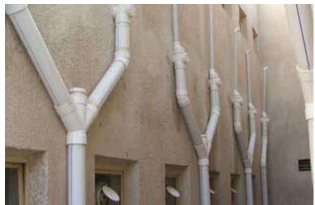
Site Photo 9. Reworked drain lines with upgraded material and improved "Y" design.
