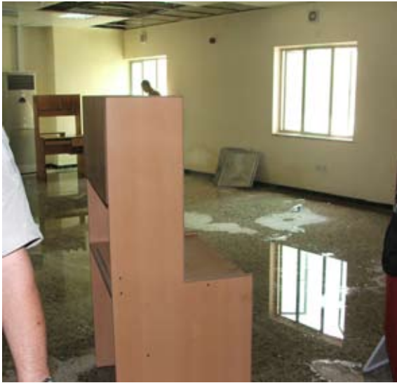
Site Photo 33. Water damage from leaking ceiling.
