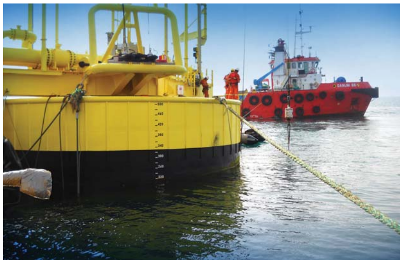
New single-point mooring facilities being installed off al-Faw Peninsula are expected to start increasing Iraq’s crude oil export capacity in 2012. (Leighton Offshore photo)
