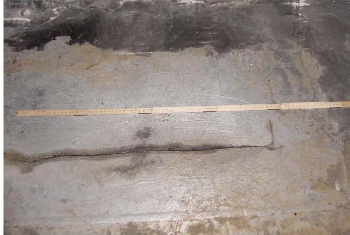
Figure 8-5 The Deck Plate Crack is Verified after Removal of Asphalt Layer (de Jong, 2006)
