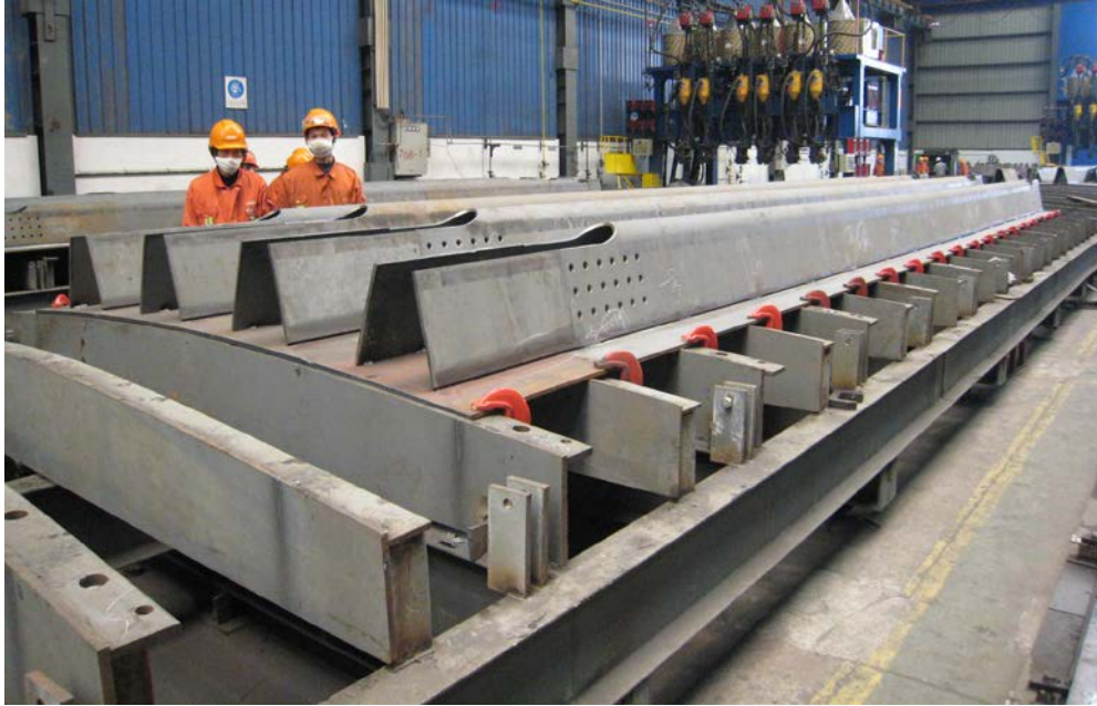
Figure 7-3 Pre-bending by Clamping the OSD to a Curved Assembly Bed is used to Offset Deck Panel Distortion due to Welding
