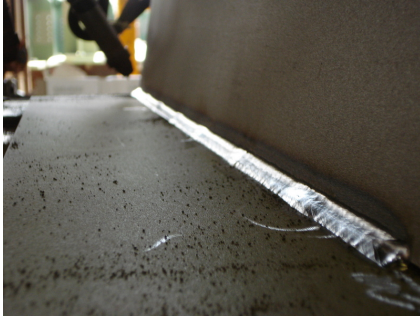
Figure 7-10 The Tack Welds Under this Cover Pass Were Re-melted, Yet Their Location is Still Obvious (This Condition is Acceptable because Profile Meets Code). The Larger Tack Welds Can Influence the Weld Profile
