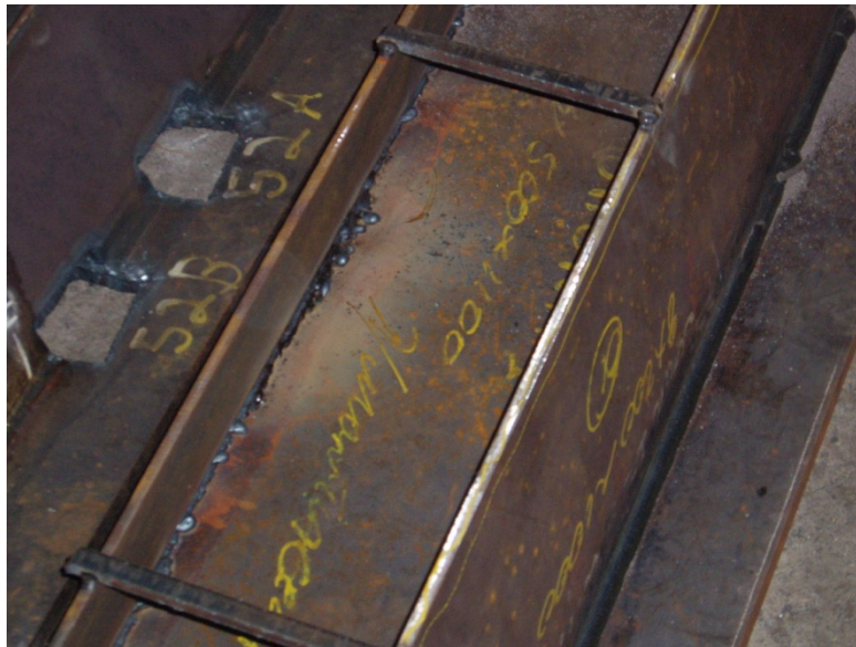
Figure 7-11 Melt-Through as Shown in this Picture is a Sign that the Joint Landing May Be Too Small
