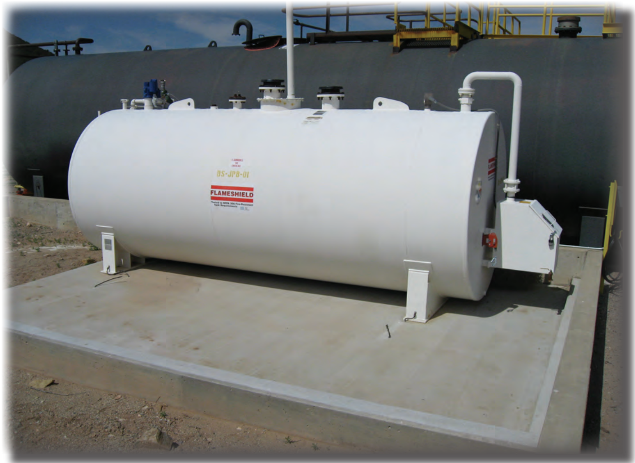
Aboveground Storage Tank
