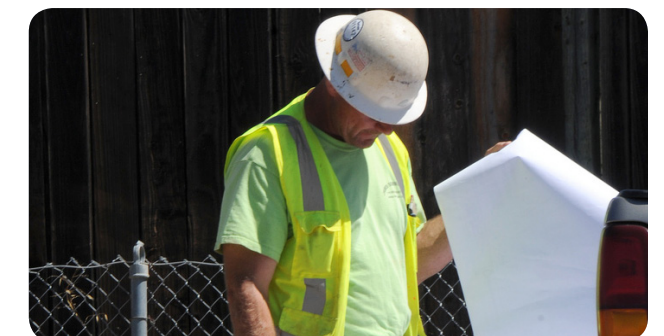
A contractor reviews the construction plans for a flood protection project in San Jose, CA.
