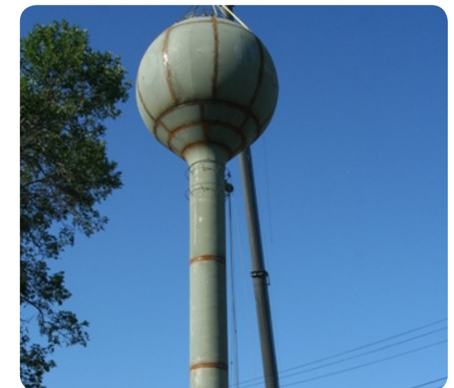
Thanks to Recovery Act funding through USDA's Water and Waste Disposal Program, a new state-of-the-art water tower will boost water pressure and improve fire safety in Ipswich, Massachusetts.
