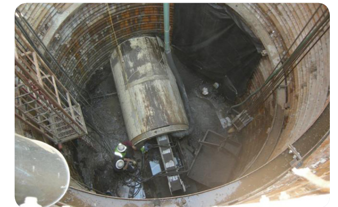
Recovery Act funding from the EPA will replace aging wastewater mains in Batesville, Arkansas. Source: EPA.
