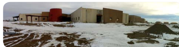
The Eagle Butte Health Center under construction in South Dakota. Source: HHS.
