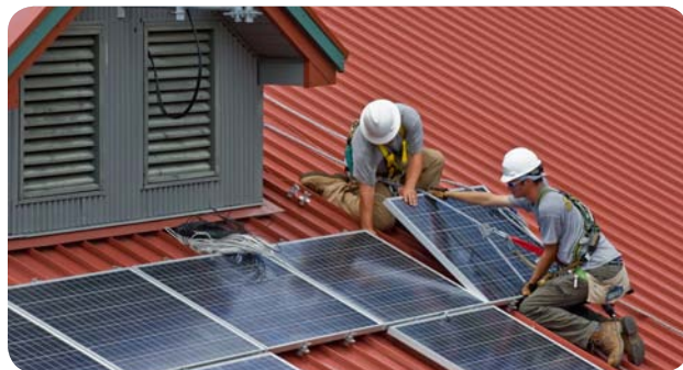
Forest Service solar panel installation. Caption: Workers install 250 Recovery Act-funded solar panels to a forest service facility in the Wayne National Forest in Ohio.
