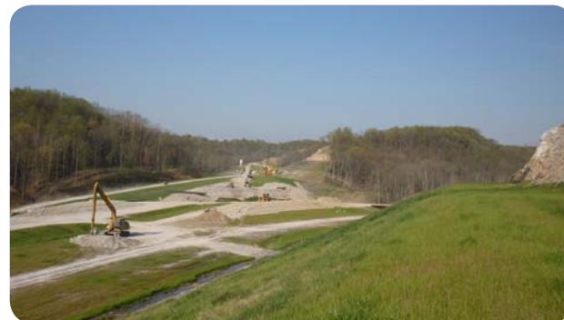
The new portion of highway to carry freight traffic in southeast Ohio under construction due to Department of Transportation Recovery Act funding. Source: DOT.
