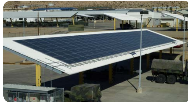
New solar panels financed through DOD Recovery Act funds will reduce energy costs for the California Marine Corps training base. Source: DOD.
