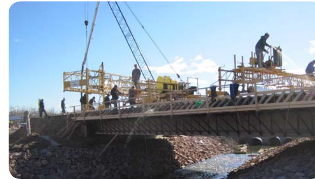
Recovery Act funding through the Department of Transportation being used to construct a bridge in South Dakota.
