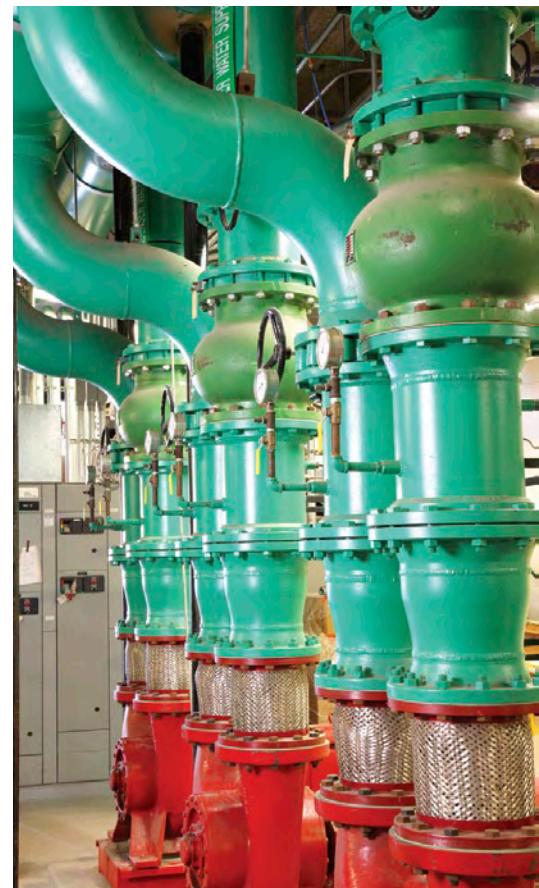
Chilled water pipes in the NCCS's mechanical room provide cooling to the center's machines.
