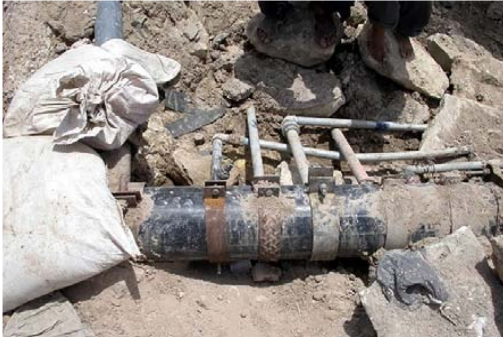
Site Photo 4. Illegal taps in the transmission and distribution lines, which reduce the water pressure and amount of water available to residents (Courtesy of USAID)
