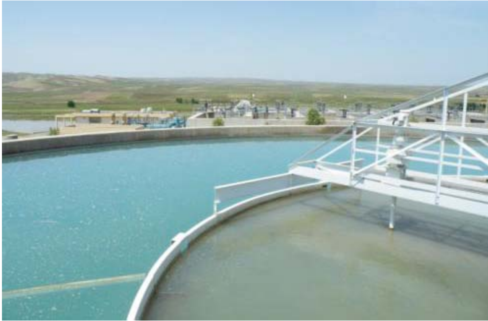
Site Photo 6. Partial view of clarifier's mechanical scraper directly settled solids to the center for disposal
