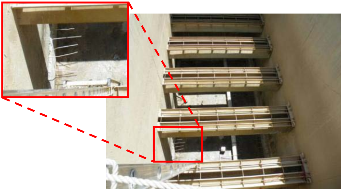
Site Photo 10. Filter with media and failed slab removed
