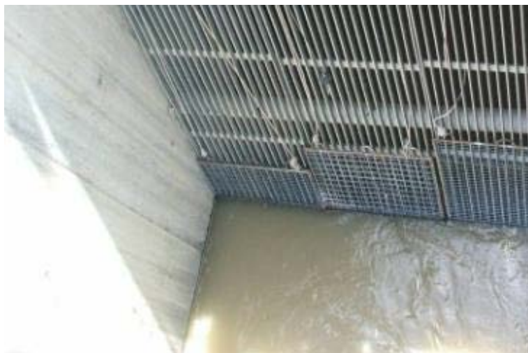
Site Photo 7. Bar screen with modifications
