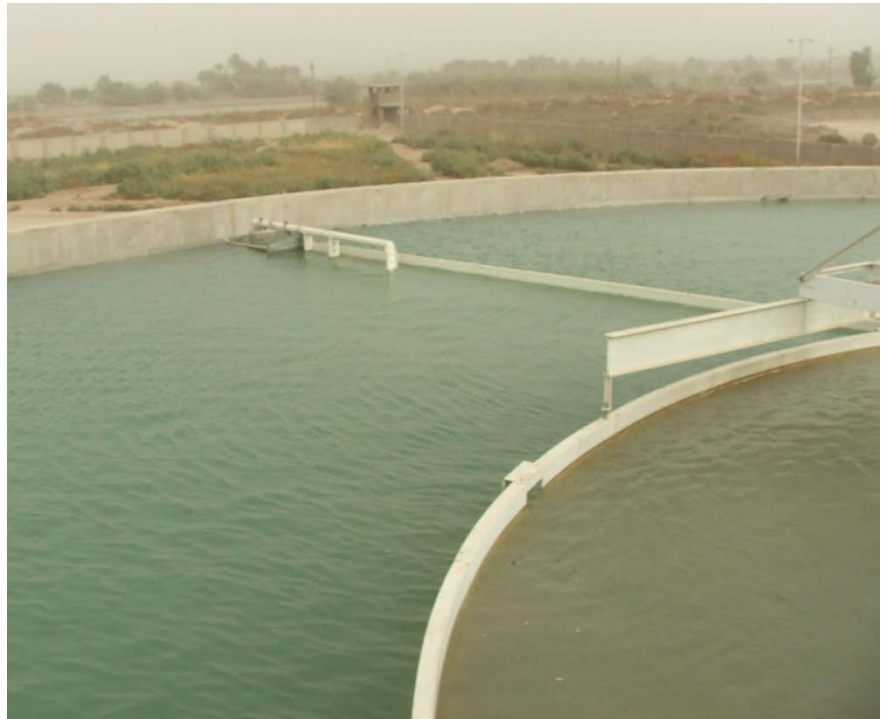
Site Photo 2. Clarifier from December 2007 SIGIR visit
