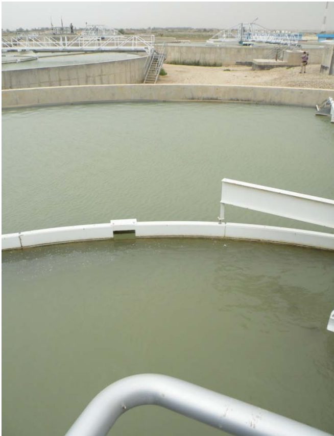
Site Photo 1. Operating clarifiers
