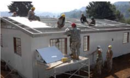
U.S. and Guatemalan Army Soldiers work on the roof of a clinic being constructed in San Marcos, Guatemala, 19 April 2007, during exercise New Horizons-Guatemala 2007. (U.S. Army photo by Juan Torres-Diaz)
