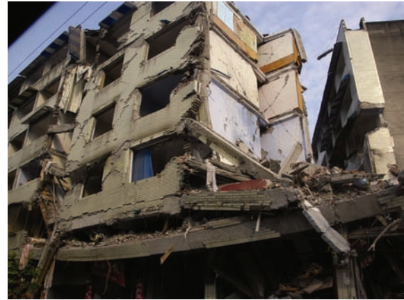
Figure 6. Partially collapsed six-story residential building (with commercial ground floor) in city of Dujiangyan, Sichuan Province, P.R. China. Collapse attributed to several factors, including poorly confined (and possibly nonductile) concrete columns and beams, lack of continuity of prefabricated floor slab diaphragms, and underestimated seismic design levels. Photo taken on August 4, 2008. Image courtesy of the Earthquake Engineering Research Institute. © 2008 by Marshall Lew.
