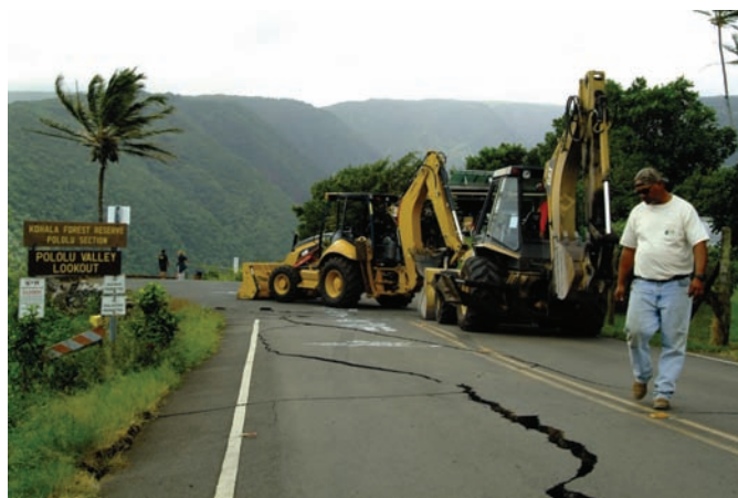
Figure 9. Kapaau, HI, October 25, 2006 – A repair crew examines the Polou Valley Lookout road, which was closed due to earthquake damage. Image courtesy of FEMA.
