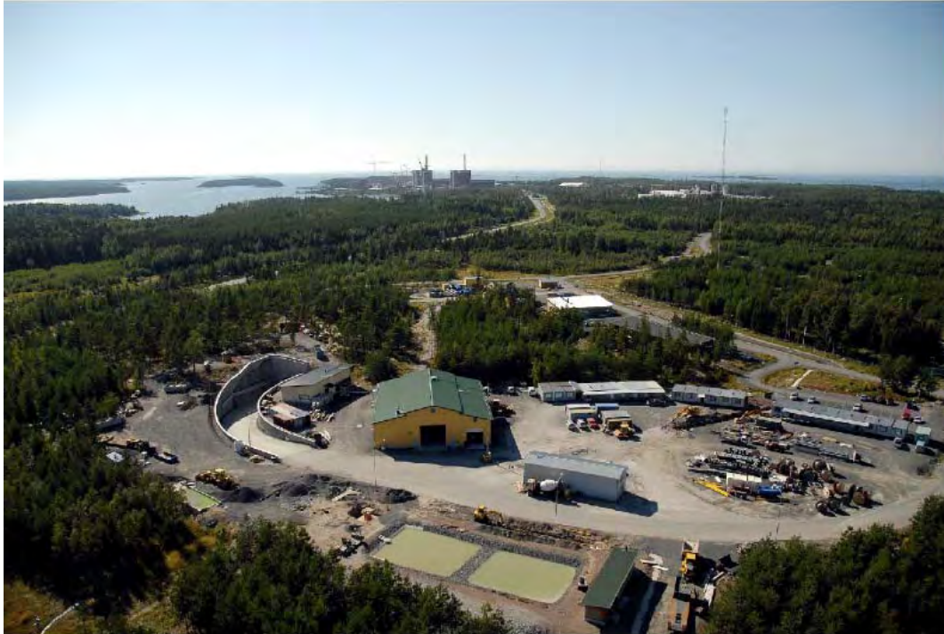
Figure 5-13 Access tunnel to the disposal facility for irradiated nuclear fuel under construction at Olkiluoto (STUK, 2008). Used with permission of STUK.
