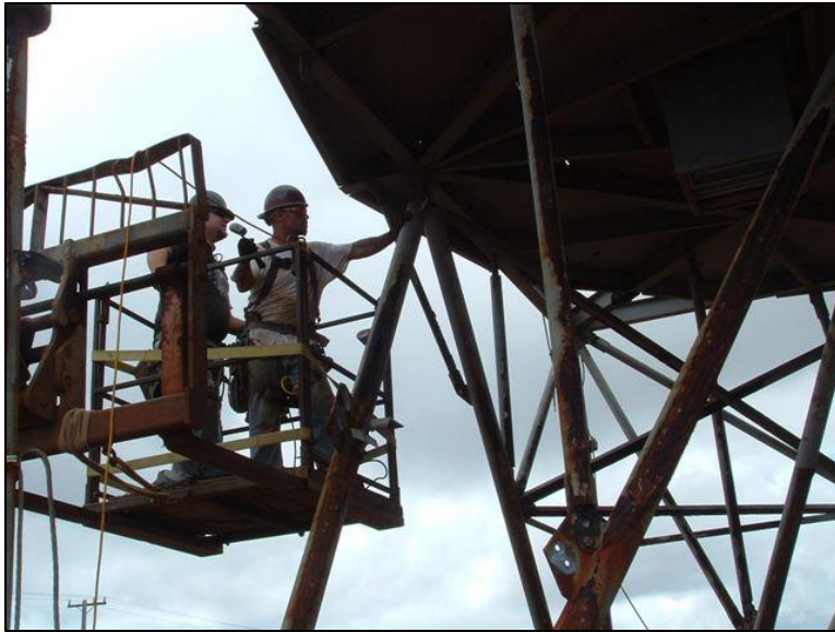
Workers begin removing the dome from the old tower...note the severe corrosion on the tower supports
