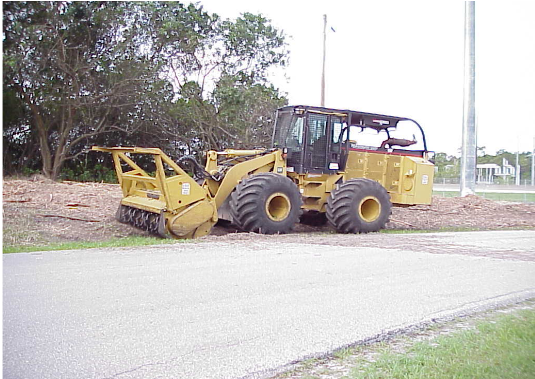
Figure 18. Front end loader in Port St. Lucie fitted with cutting/grinding attachment for removal of Brazilian peppertrees along roadside rights-of-way (Photo credit: J. Dunton).
