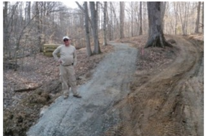
BLM trail builder David Lyster, hired with ARRA funds, on a relocated section of a trail. The old trail, at right, will be removed and landscaped.
