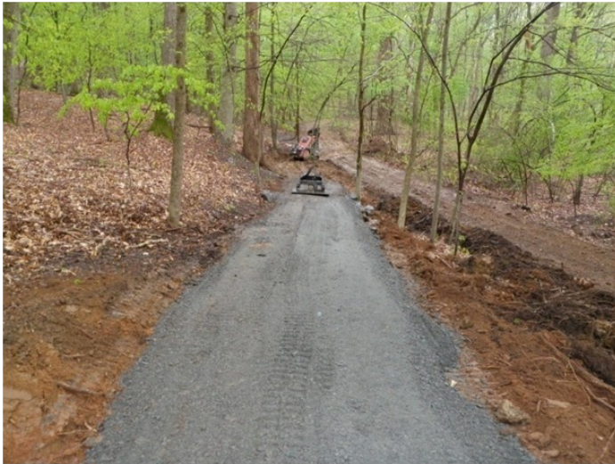
The original poorly-drained trail on the right is being relocated to the left.
