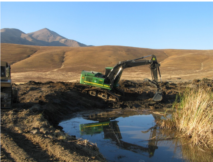
An equipment operator uses an excavator to restore habitat on one of the ponds.
