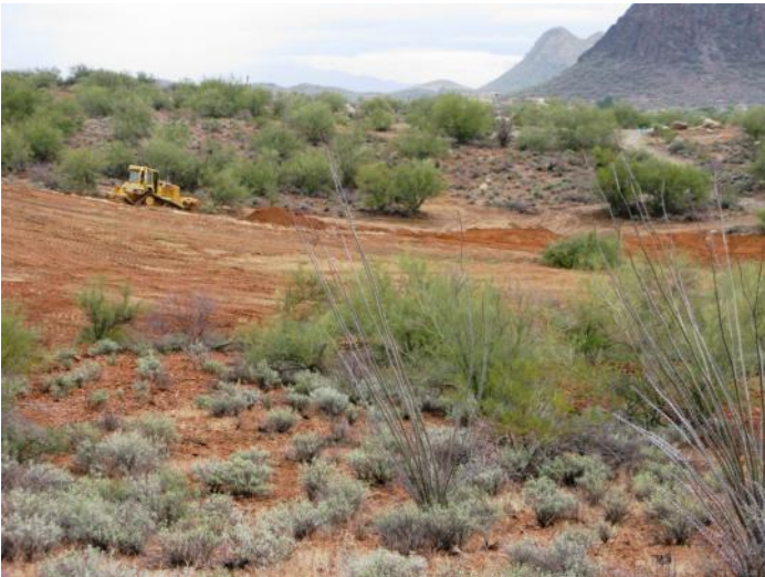
This former mine site near Tucson, Ariz., is among those being evaluated in the Restoration Design Energy Project.
