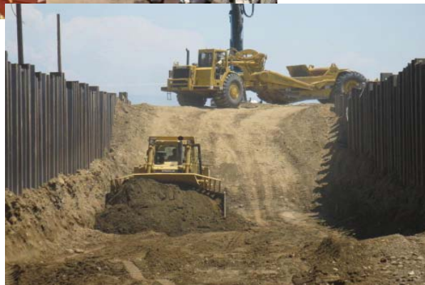
Heavy equipment excavates the canal on the east side of Red Bank Creek.
