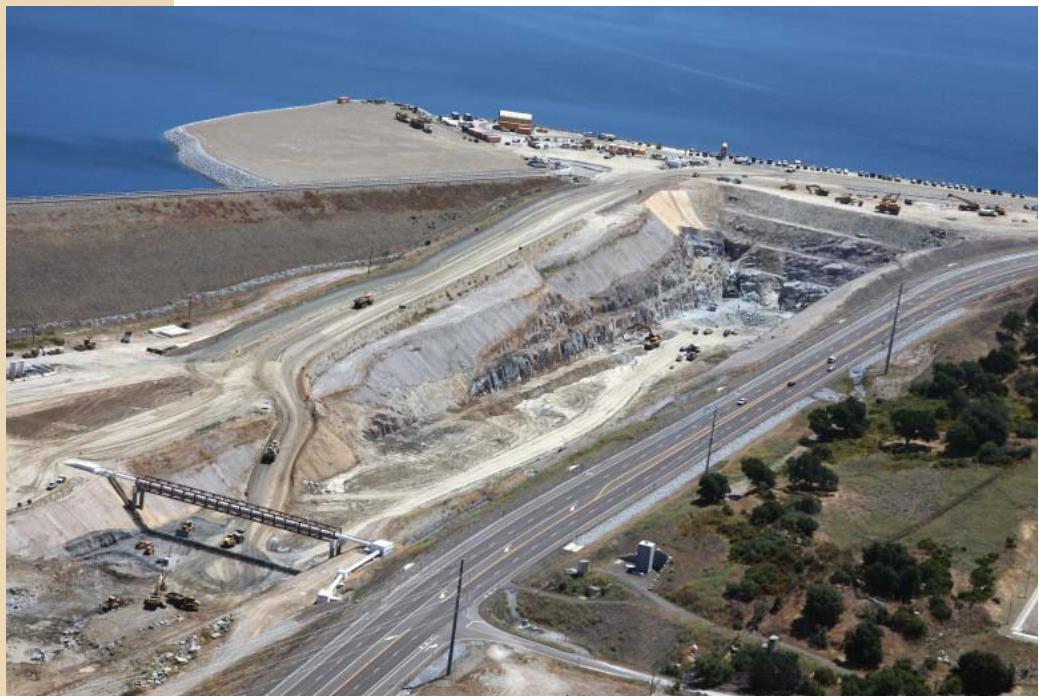
View of upper auxiliary spillway, expanded overlook area, and Natoma pipeline bridge in the foreground.
