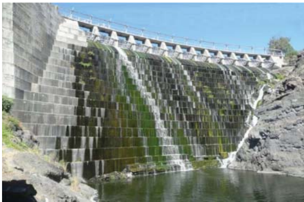
Copco 1 Dam, which is 115 feet in height, is another of the dams that may be removed from the Klamath River.
