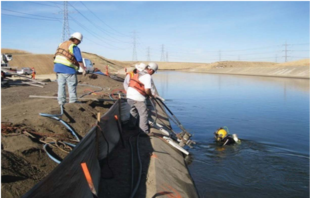
Diver begins cutting canal's concrete liner in the first stages of the project.
