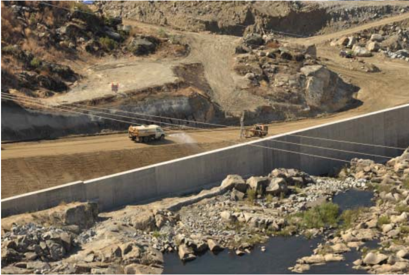
A view of the lower stilling basin access road and cofferdam wall.
