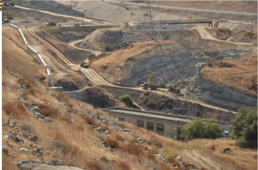
Contractors build an access road to the new auxiliary spillway, with a new pipeline shown at left.
