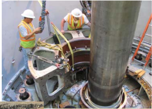
Contractors remove a turbine bearing as part of the hydroelectric plant overhaul.
