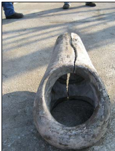
Failed Mooring Socket
