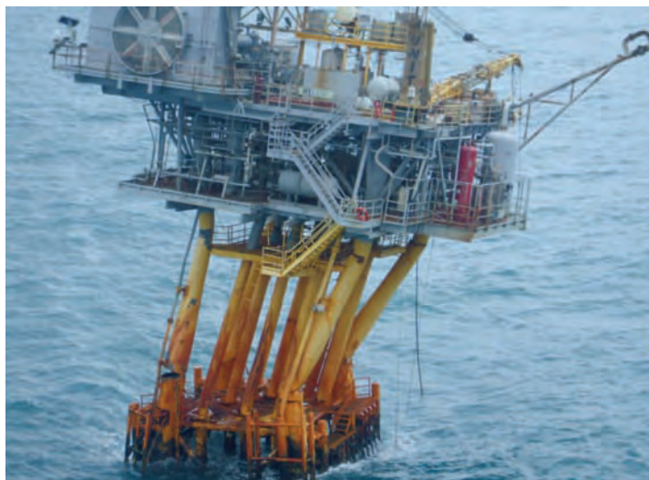
A platform with wave-in-deck damage.
