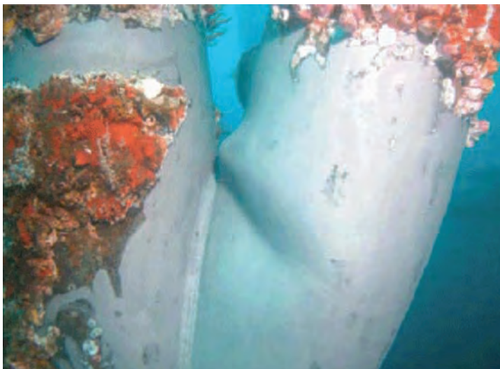
A buckled underwater brace of a platform.
