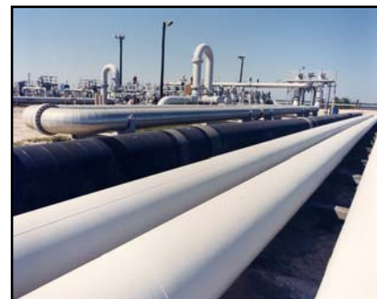
Bryan Mound SPR site Photo provided by the U.S. Department of Energy
