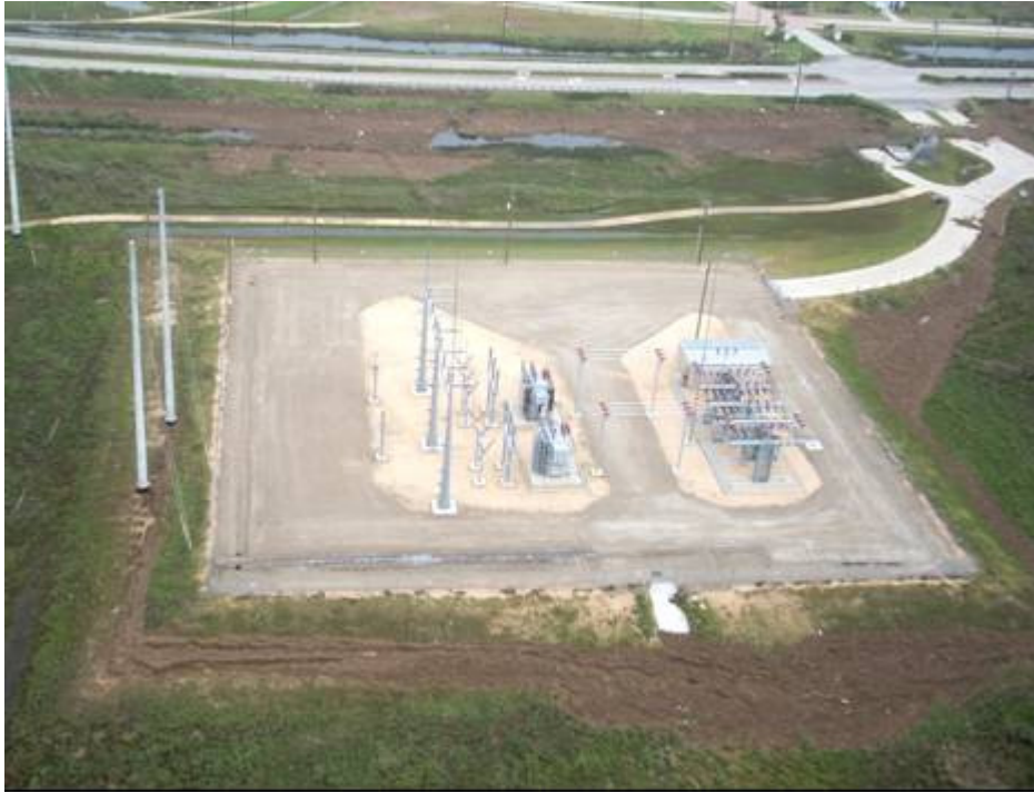
Figure 5-1. CenterPoint's West Bay Substation.
