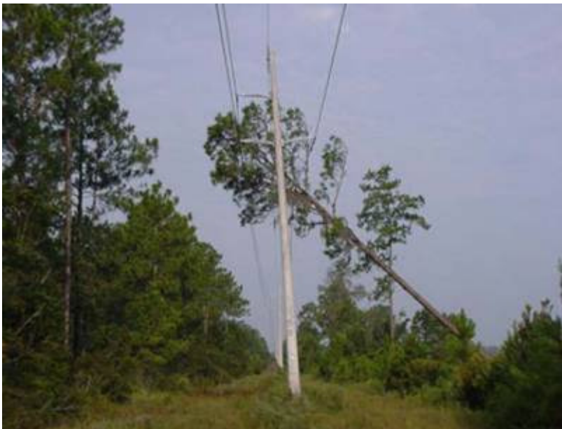
Figure 3-1. Tree falling into transmission lines.
