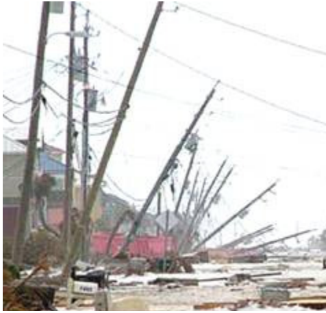
Overhead lines damaged in a coastal area.
