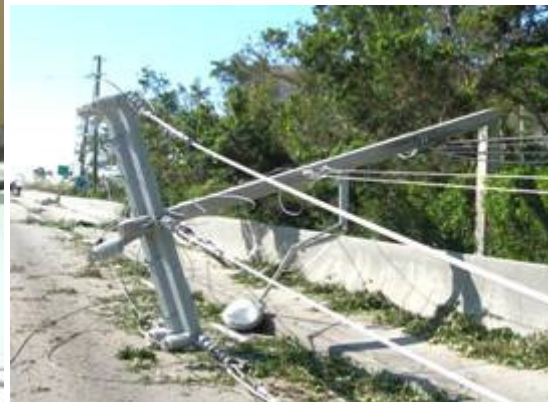
A concrete pole broken by high winds.
