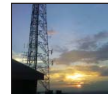
Telecommunications tower atop Ranger Peak.
