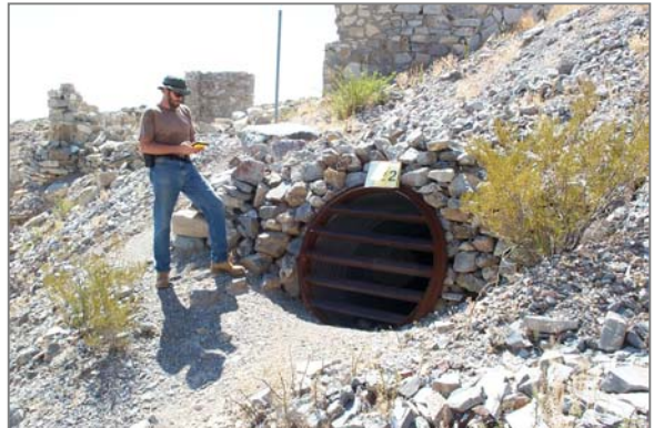
Big Bend National Park - adit with angle-iron bat gate closure
