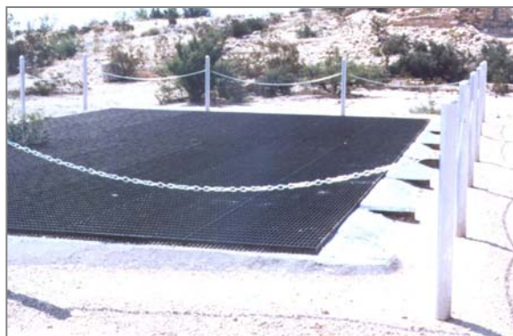
Terlingua mine shaft with steel grate closure
