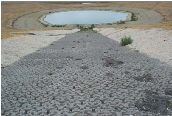
Interlocking blocks are sometimes used to armor drainage channels and establish erosion control.
