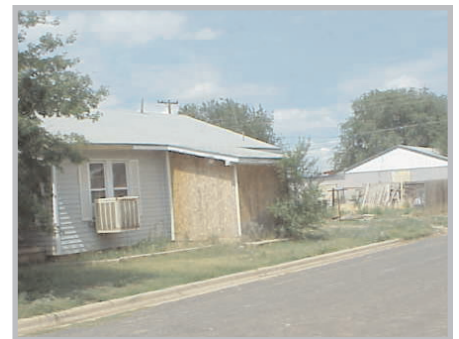
HOUSING IN NEED OF REHAB
