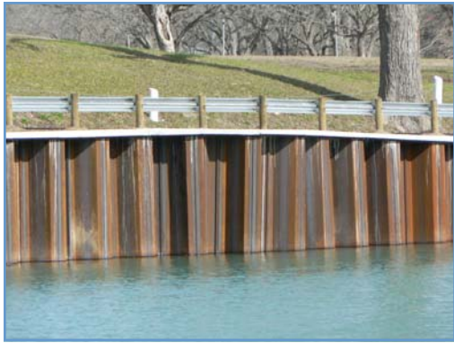
Sheet piling was installed during the Bank Stabilization Project on River Road Drive in Max Starcke Park West.
