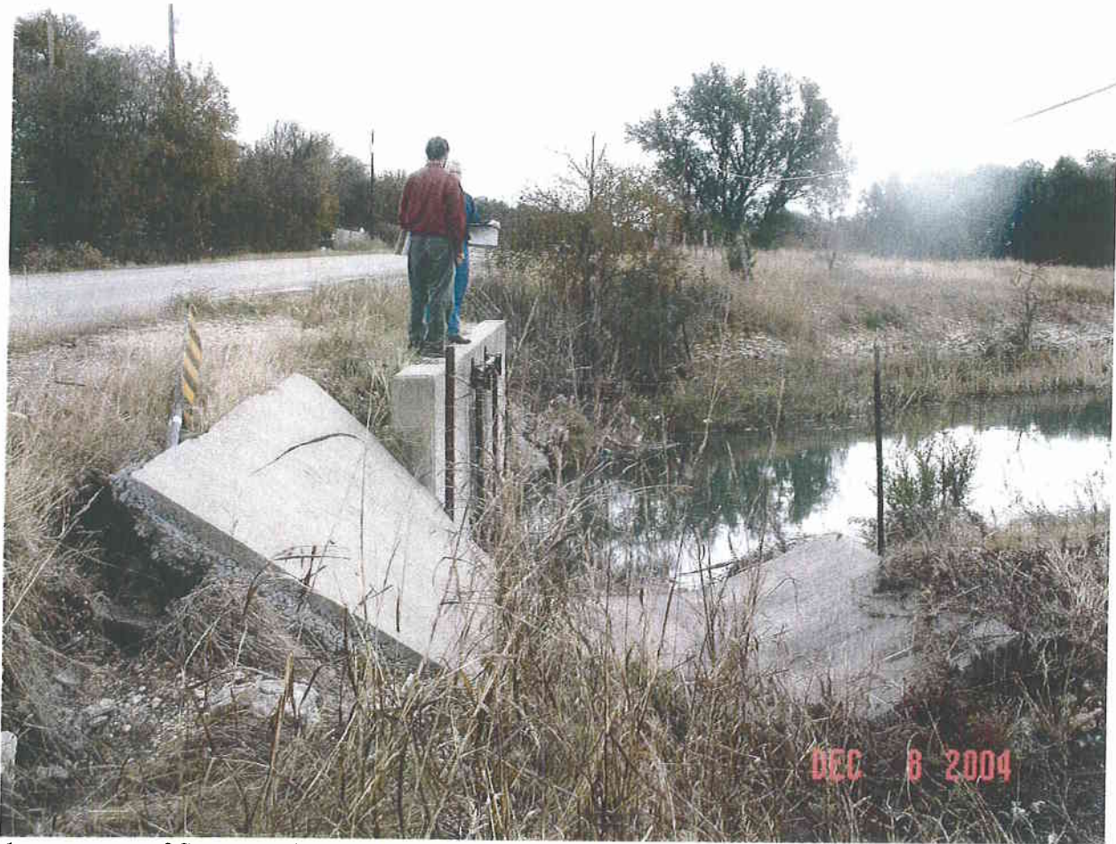
downstream of Stagecoach Rd, concrete apron erosion from roadside ditch
