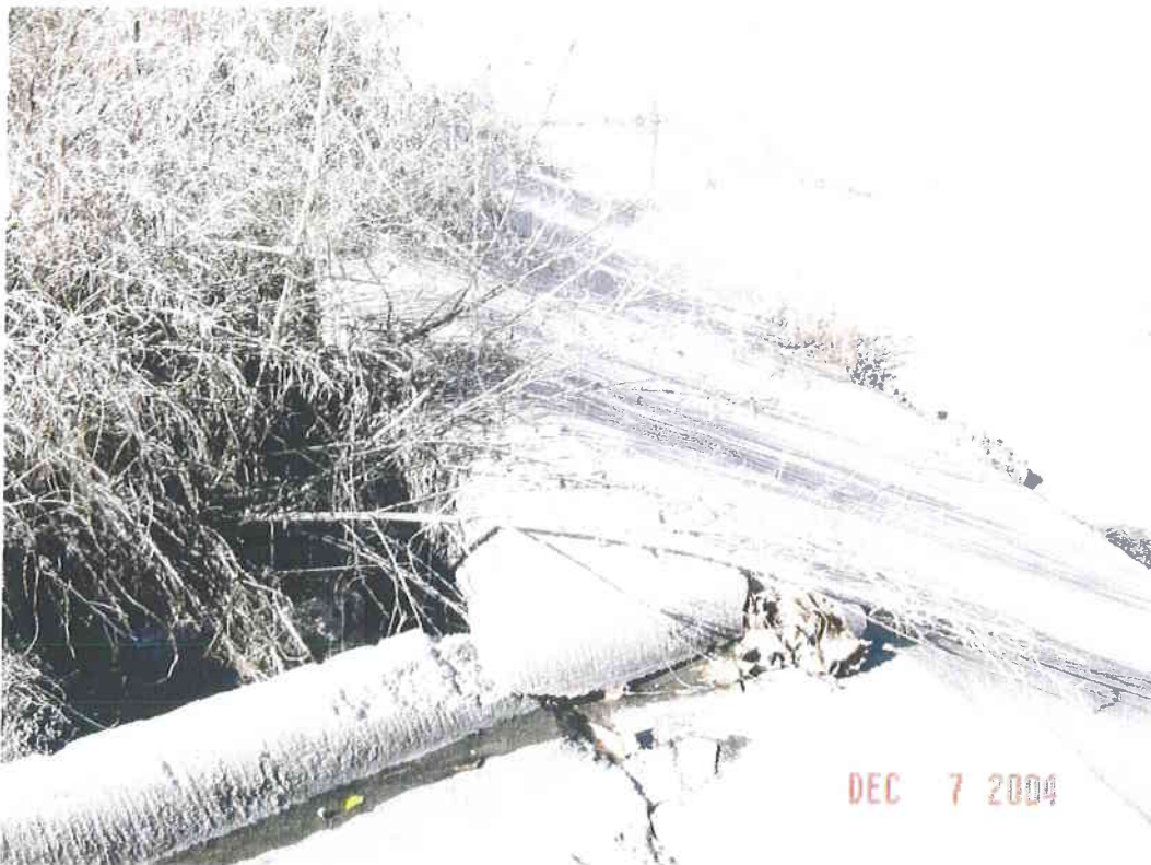
At Janice Street Downstream view of cracks in concrete channel
