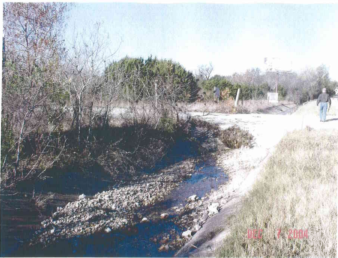
Debris and gravel accumulation upstream of driveway culvert
