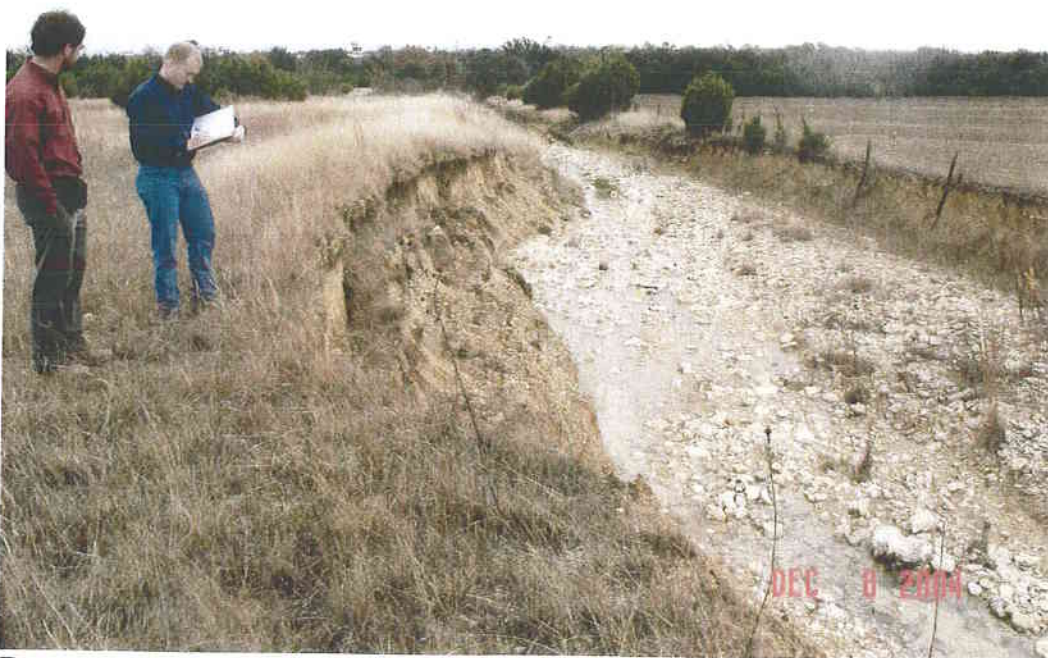
Downstream view of bank cutting or falling off
