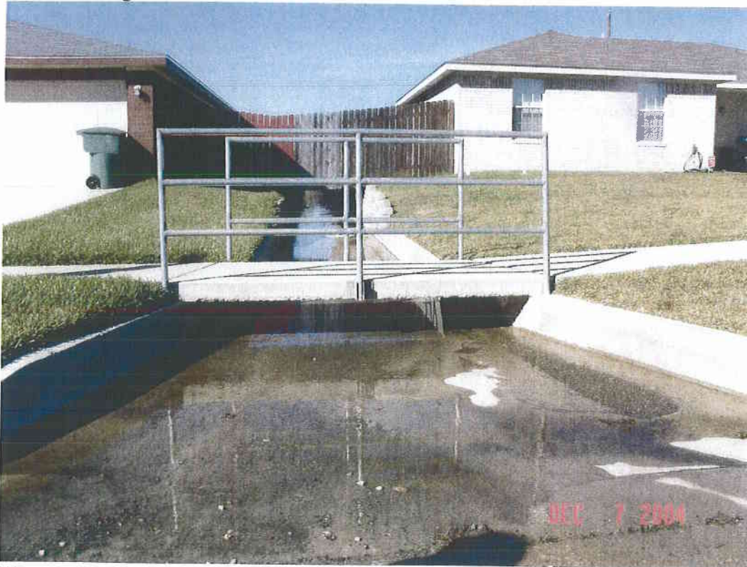
Flume at Boswell Dr, drains to Hilliard Ditch Trib.
