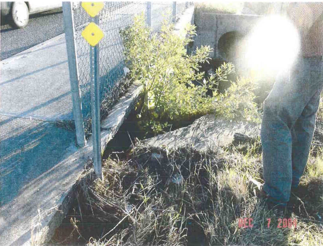
Erosion at downstream face of Rancier Ave
