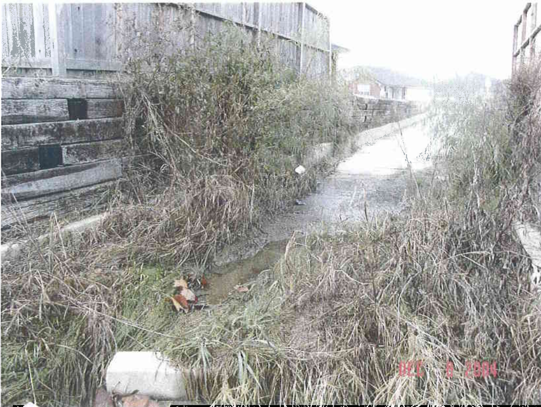
Flume into Acorn Creek just upstream of end of concrete, vegetation at the downstream outlet into the channel
