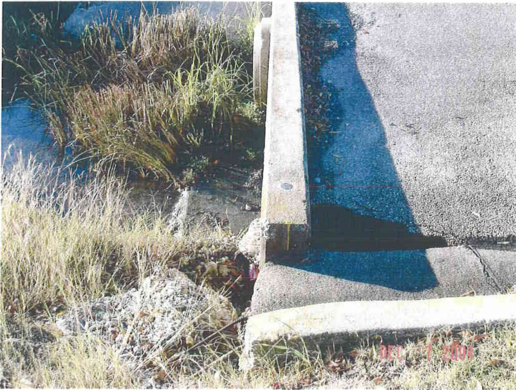
Undermining of Branch Dr at culvert
