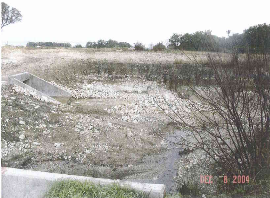
Downstream face of new Dripping Springs Dr culvert, erosion from Stillwood Dr storm sewer
