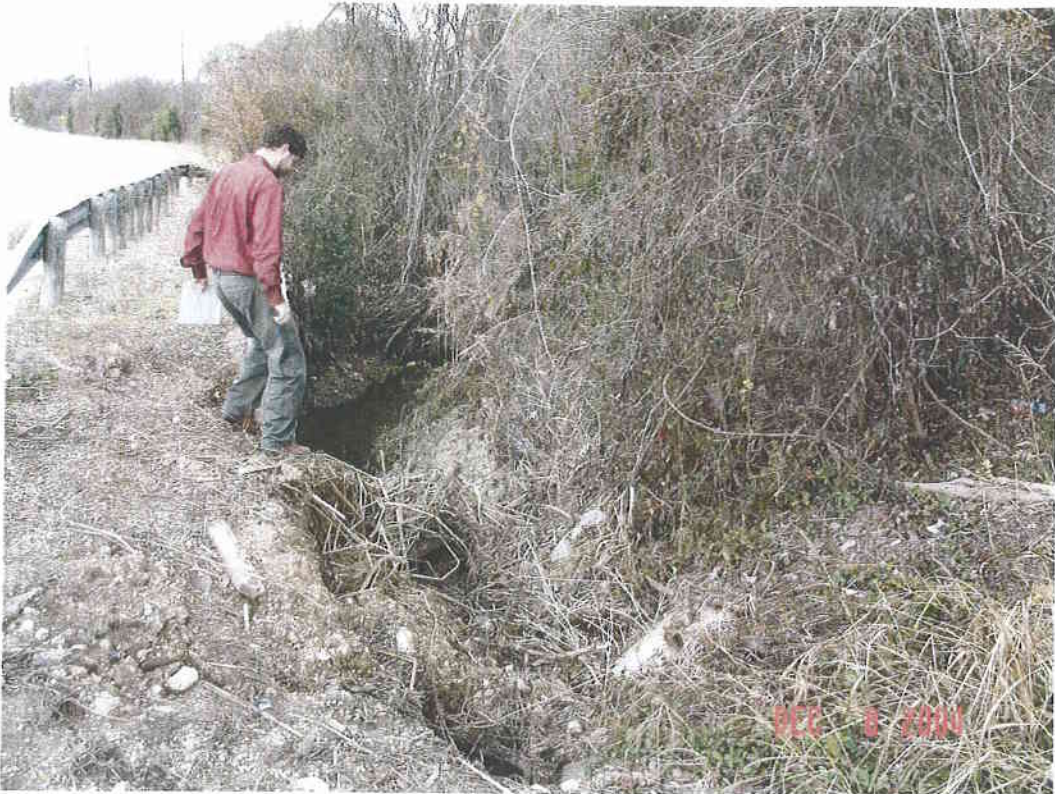
Upstream of Stagecoach Rd at Embers Ditch, erosion at northeast headwall
