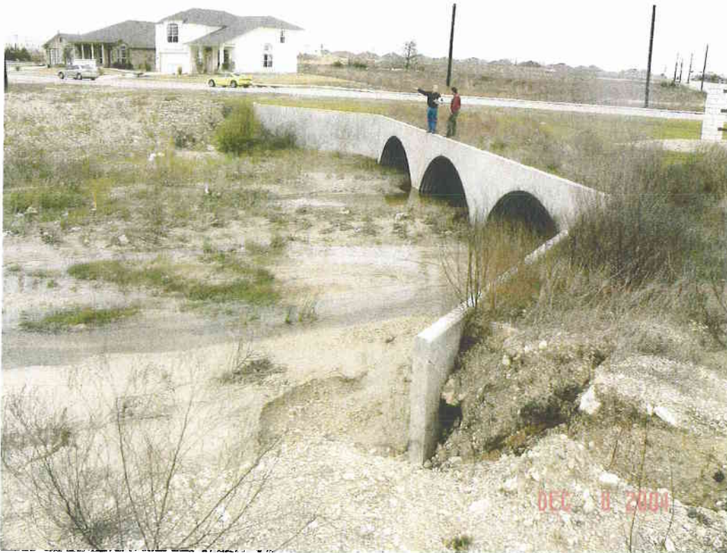
Upstream WS Young Culverts Sediment deposit, eroding wingwall
