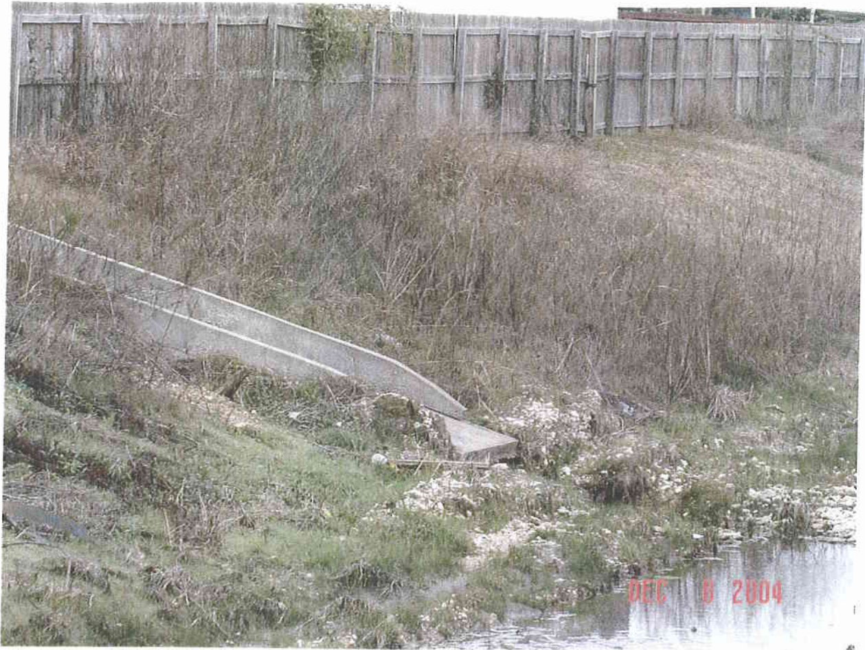
Erosion at flume from Embers Dr
