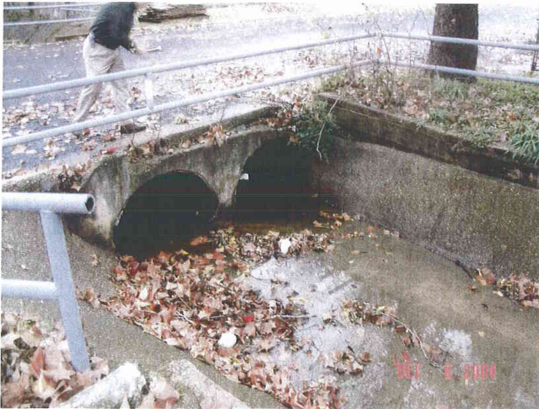
Downstream face of Wisconsin St culvert, standing water in culverts
