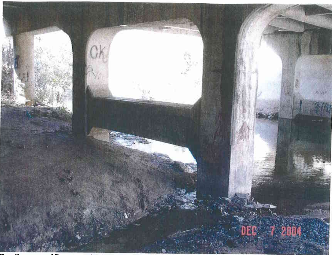
Confluence of Dogwood channel and LNC. Erosion at piers under 190
