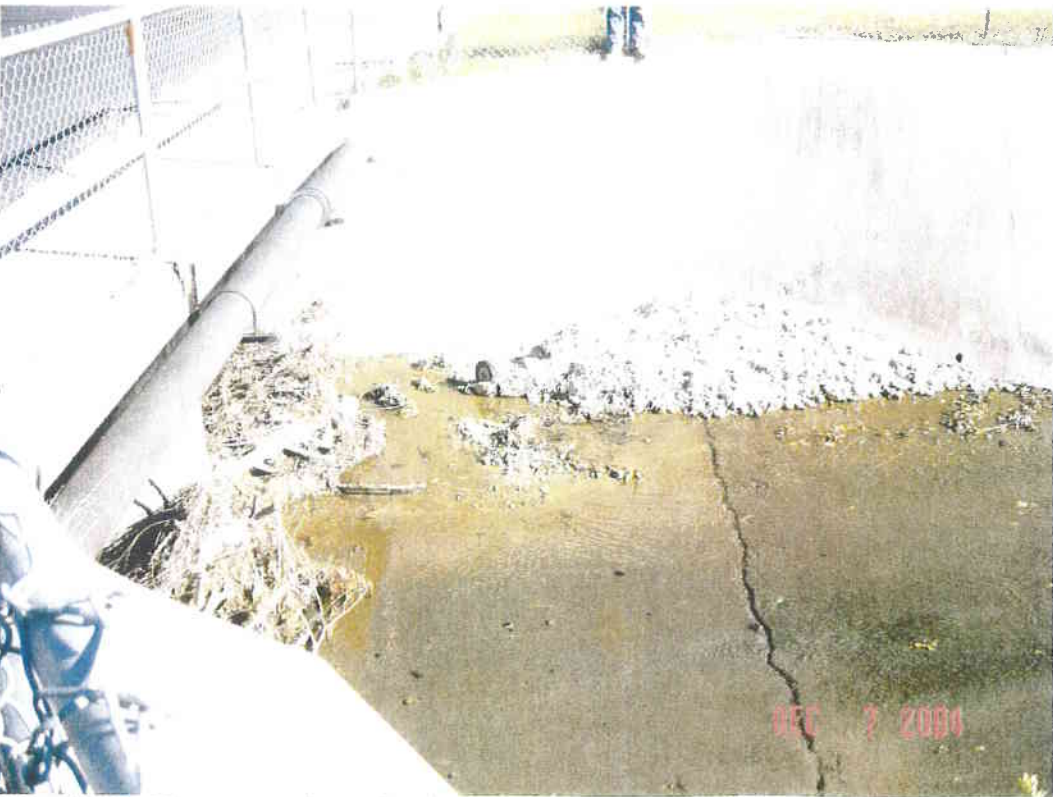
Wheeler St. Upstream view of culverts with sediment and debris
