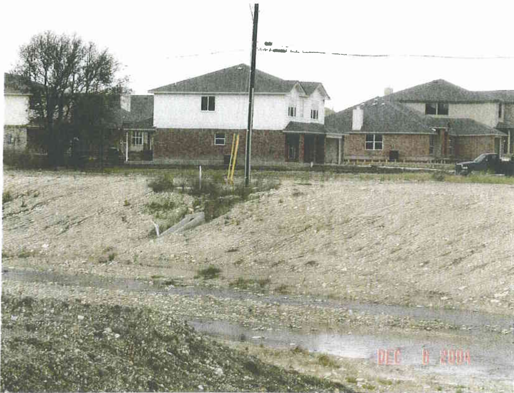
storm drain discharge undermined in channel bank
