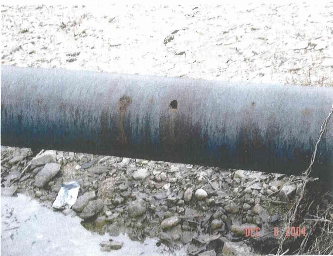
hole in sewer pipe
