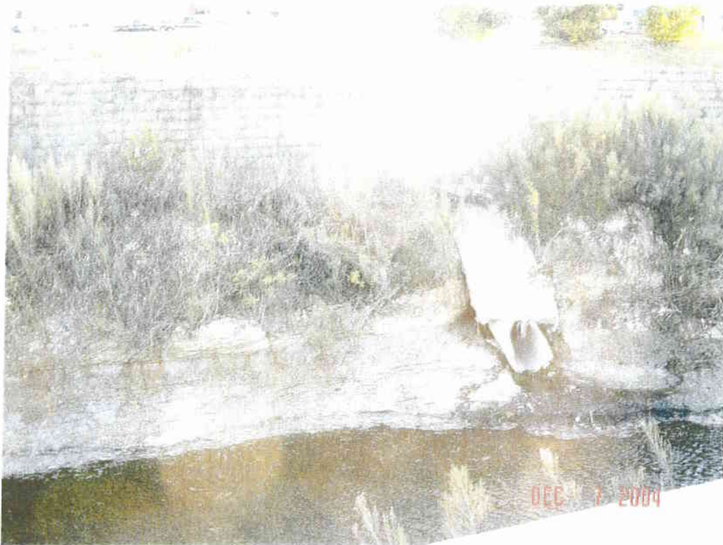
Storm sewer pipe undermined
