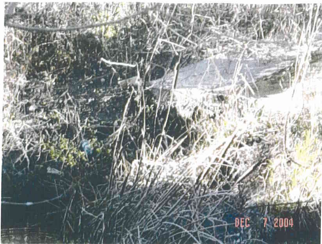
erosion at end of flume
