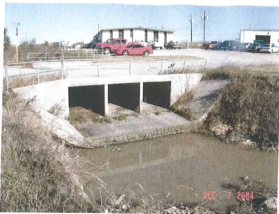
Downstream face of Jacobs Ln culvert, scour hole at end of concrete
