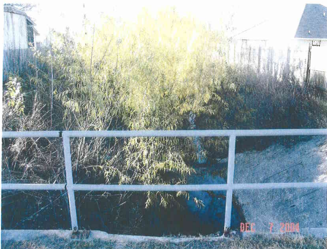
Looking downstream from Westcliff Rd, scour hole just downstream of concrete
