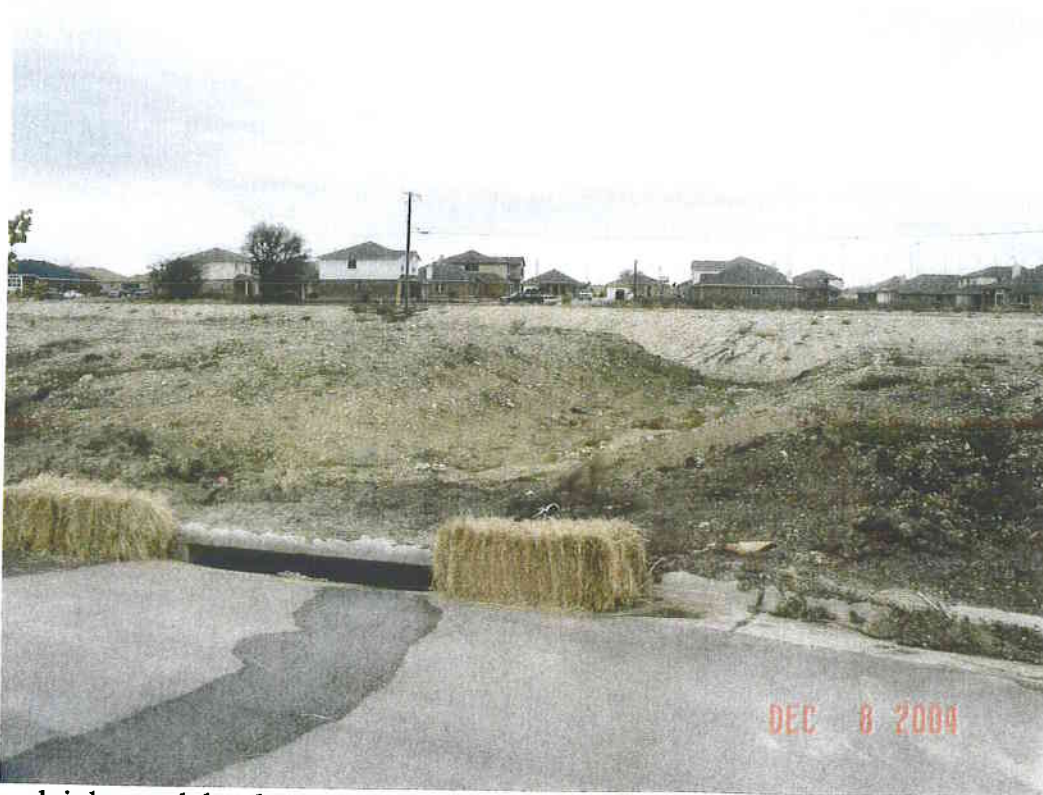
curb inlets and development area bare soil eroding
