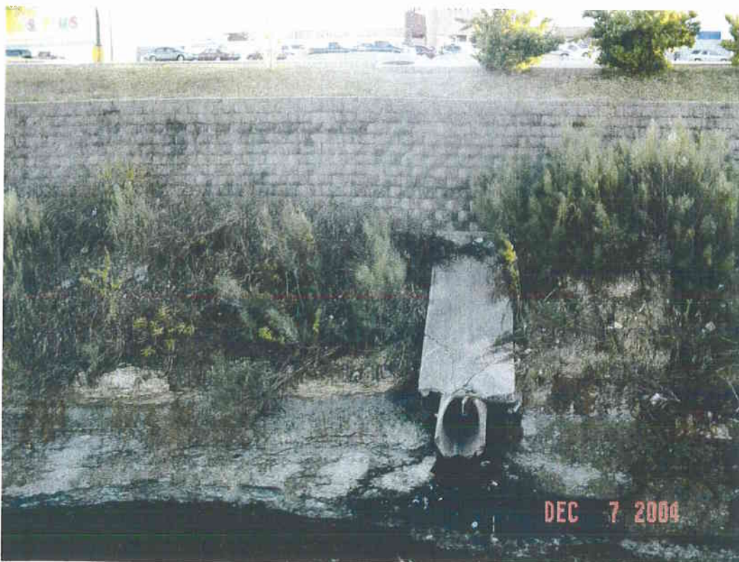
Storm sewer pipe undermined
