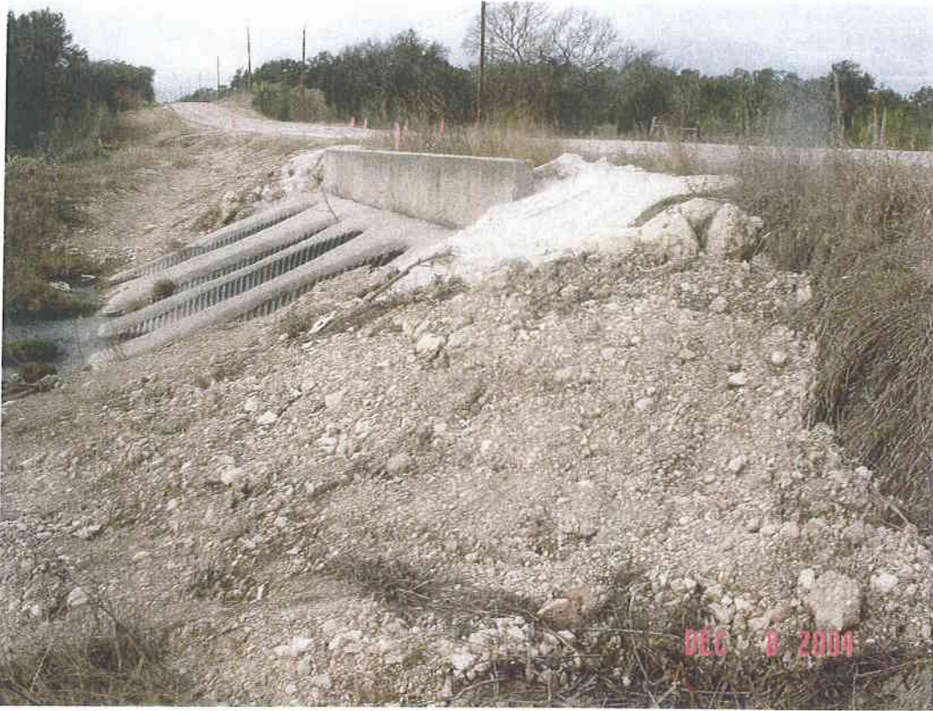
Bare soil around culvert at Stagecoach Road.
