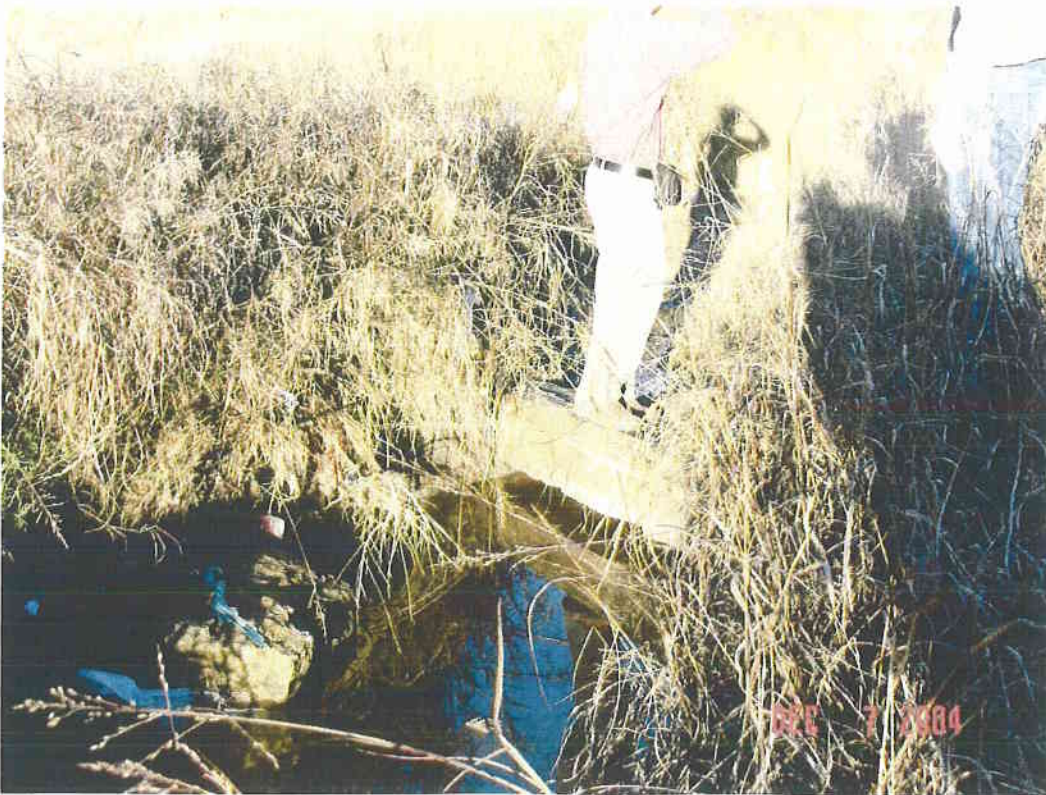
undermined drop structure
