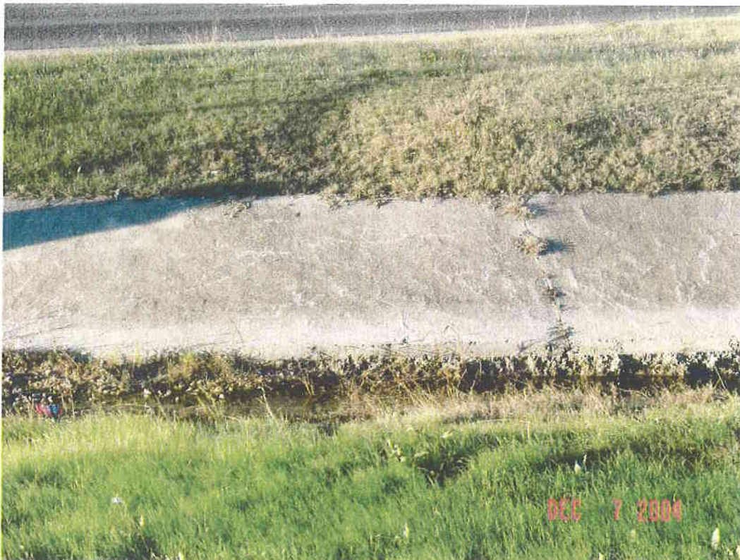
Concrete slope protection along Rancier Ave undermined
