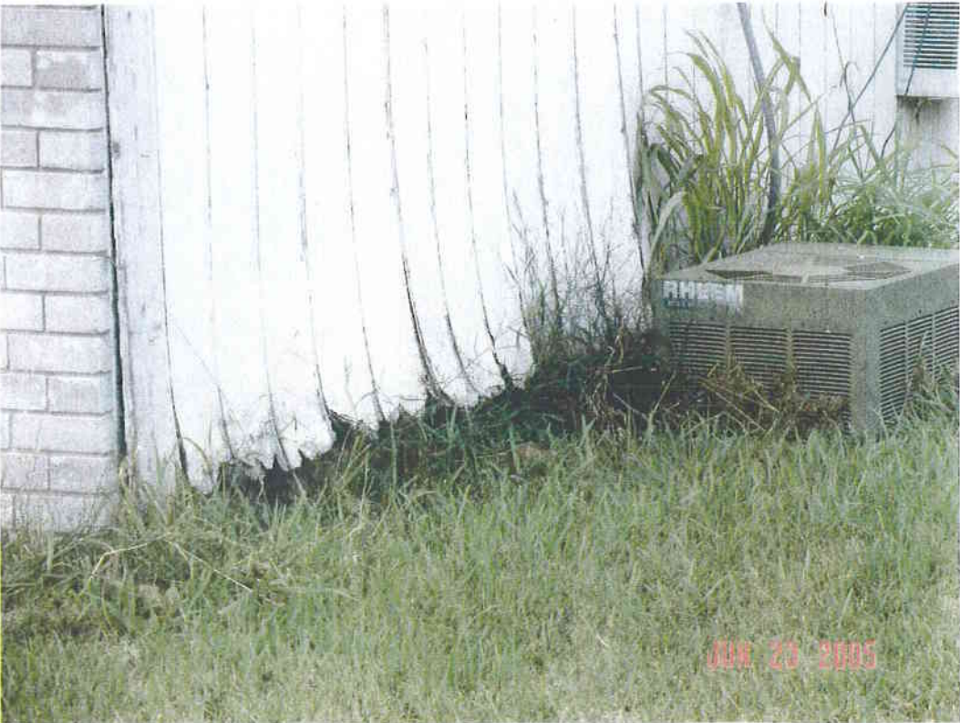
Water damage at house on Magnum Dr
