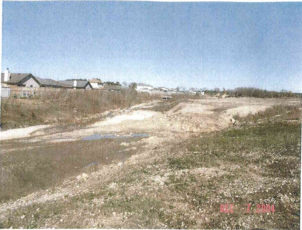
Hilliard Ditch, new development between Boswell Dr. and Blackburn Dr. Looking upstream at confluence of Hilliard Ditch and Hilliard Ditch Tributary
