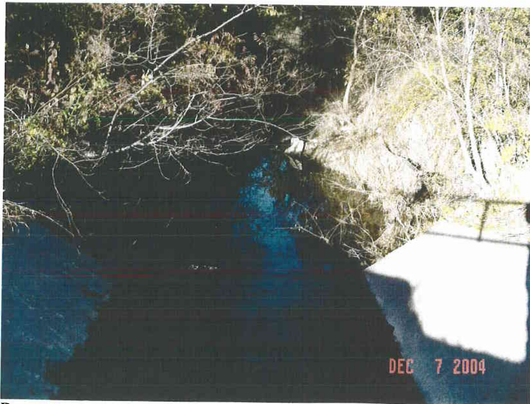
Downstream of culvert, scour hole
