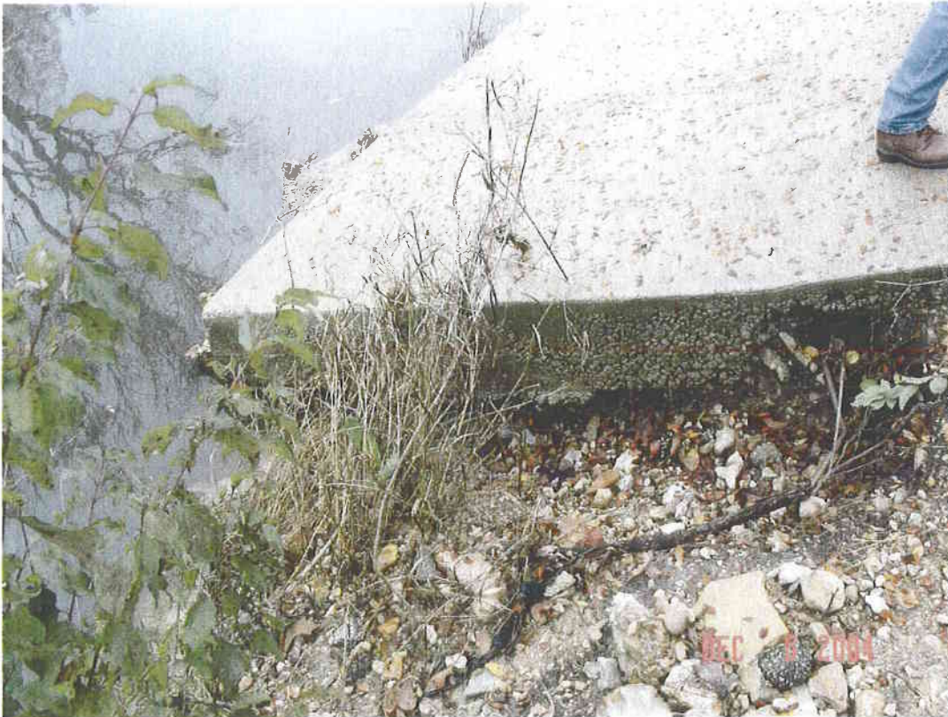
Erosion at concrete bank armoring
