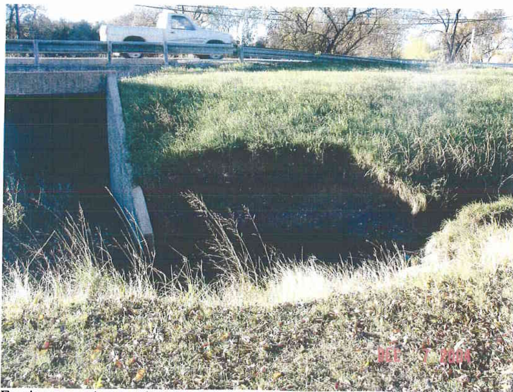
Erosion at northwest wingwall from Long Branch Tributary
