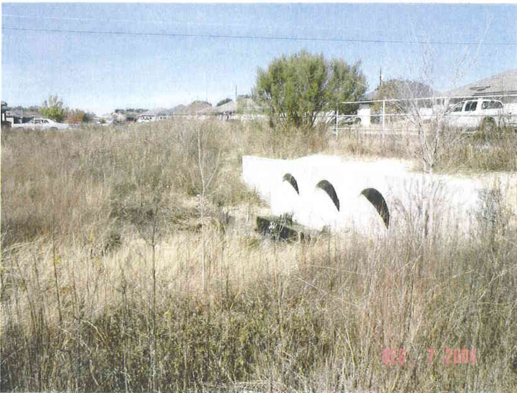
Downstream face of Ridgehaven Dr culvert, scour
