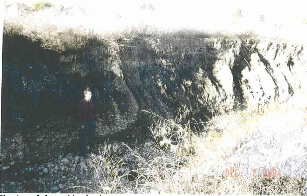
Erosion of channel banks downstream of Caprock Dr
