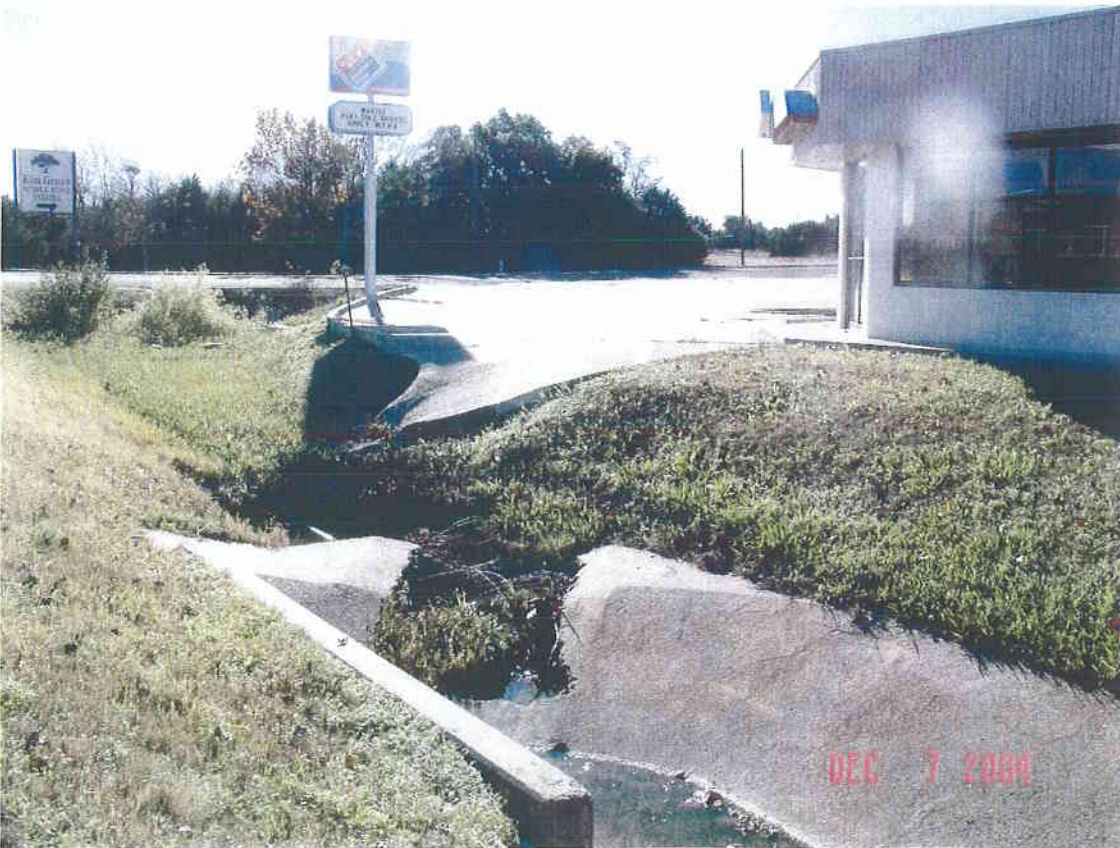
Parking lot flows through flume, discharges upstream of concrete channel. Concrete channel failure in bend.
