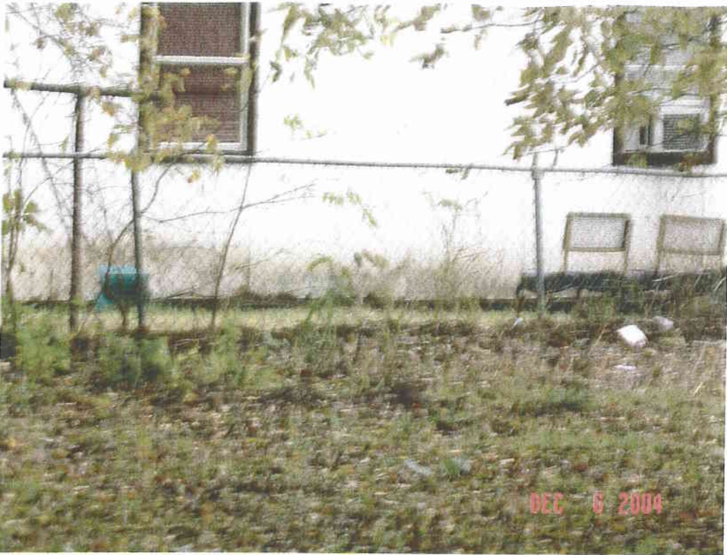
High water marks on house on Vermont Street from Utah Street flow overtopping curb and gutter
