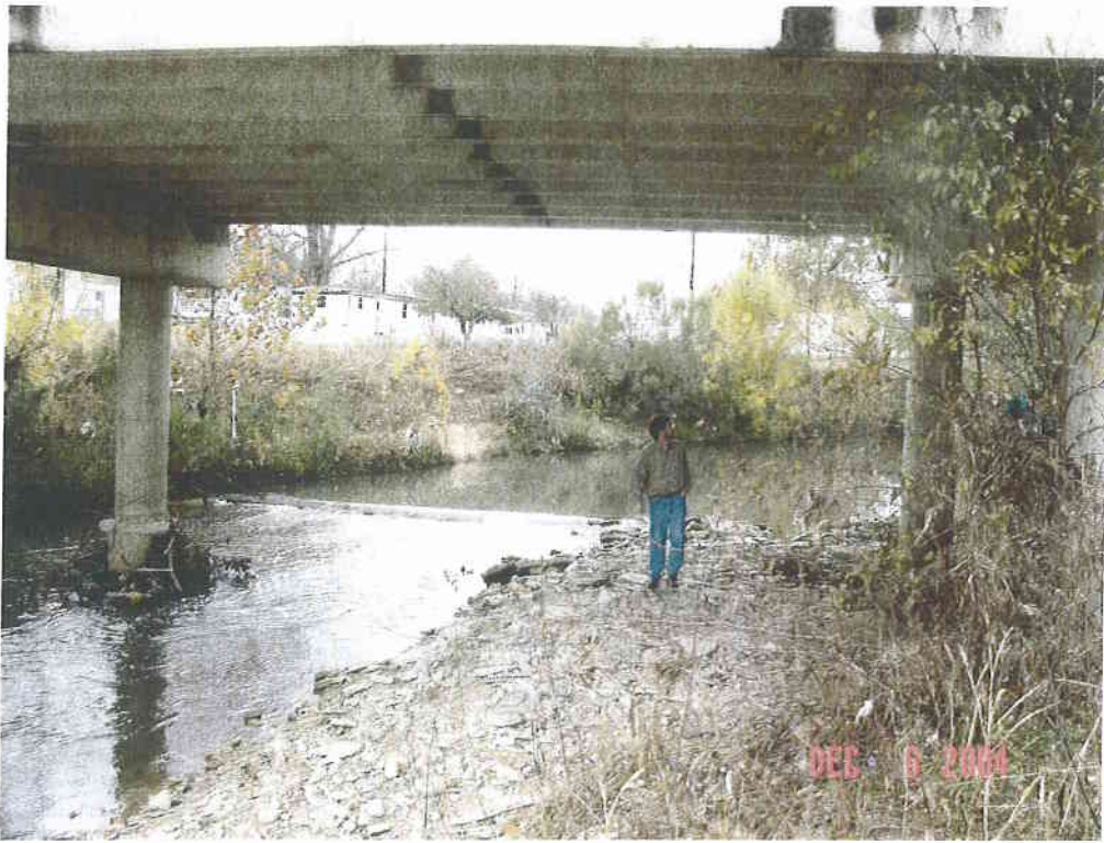
Looking downstream, bank erosion
