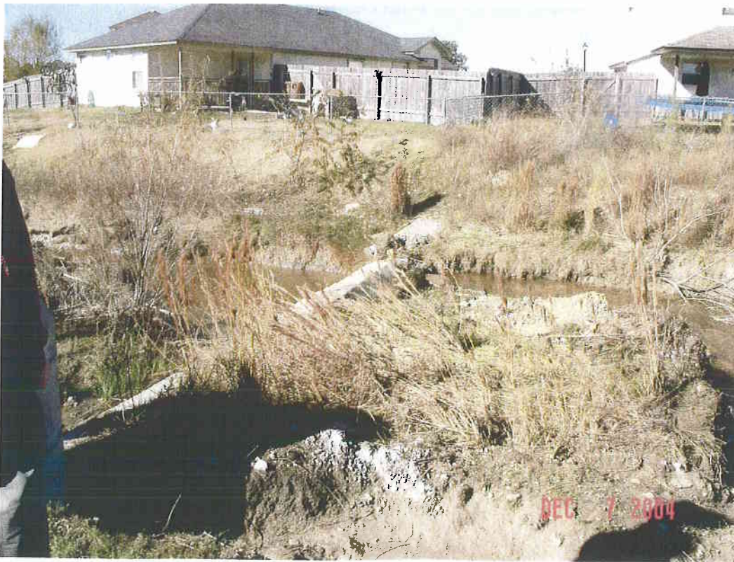
Exposed utility crossing
