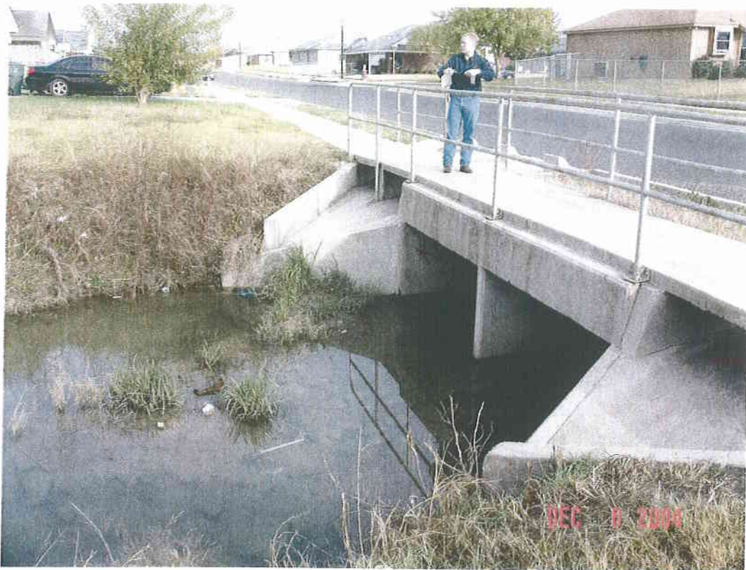
Downstream face of Water Oak Dr culvert on Embers Ditch, East Trib
