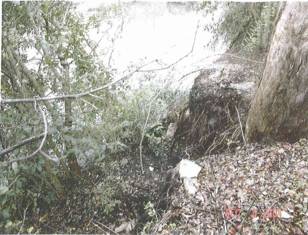
Erosion of channel bank along Odom Drive
