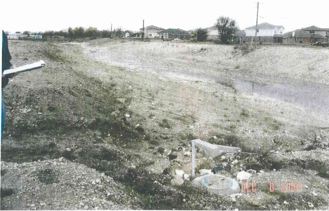
erosion from street flow, erosion around manhole and storm drain discharge
