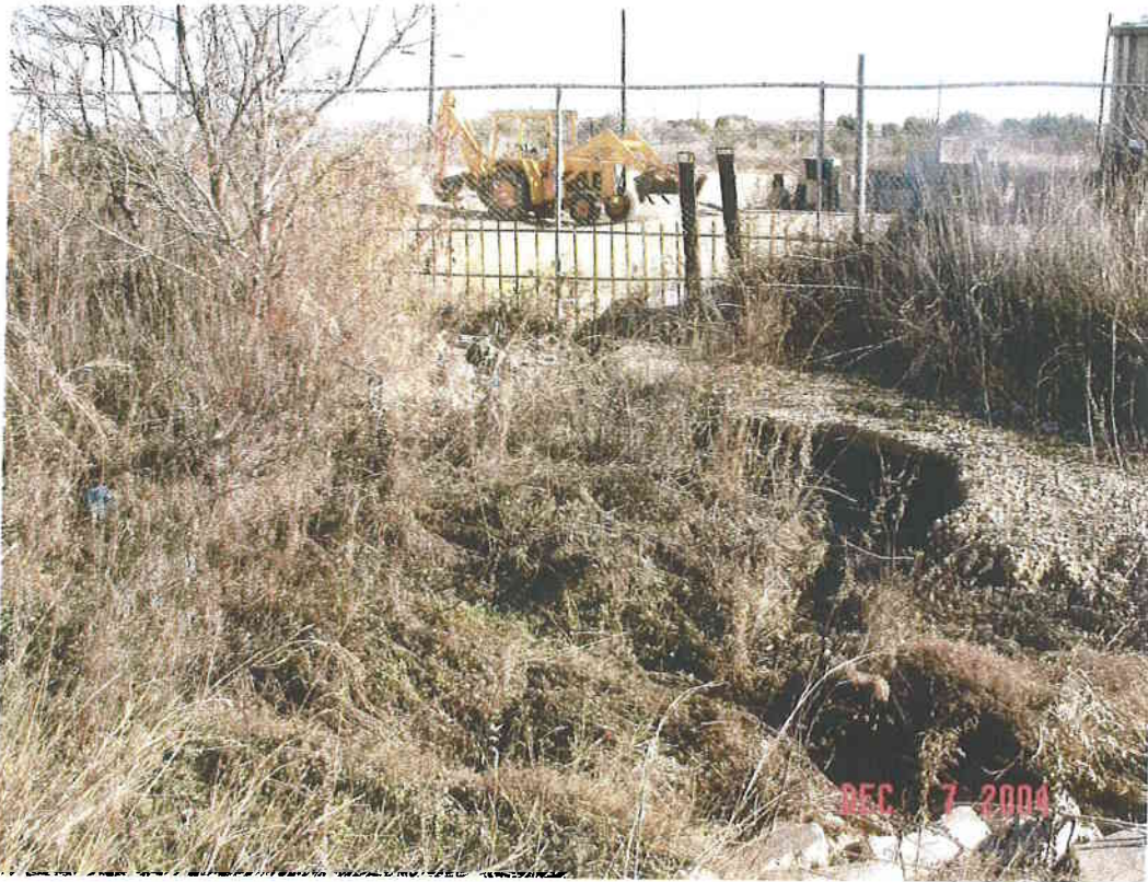
erosion from drainage off industrial yard
