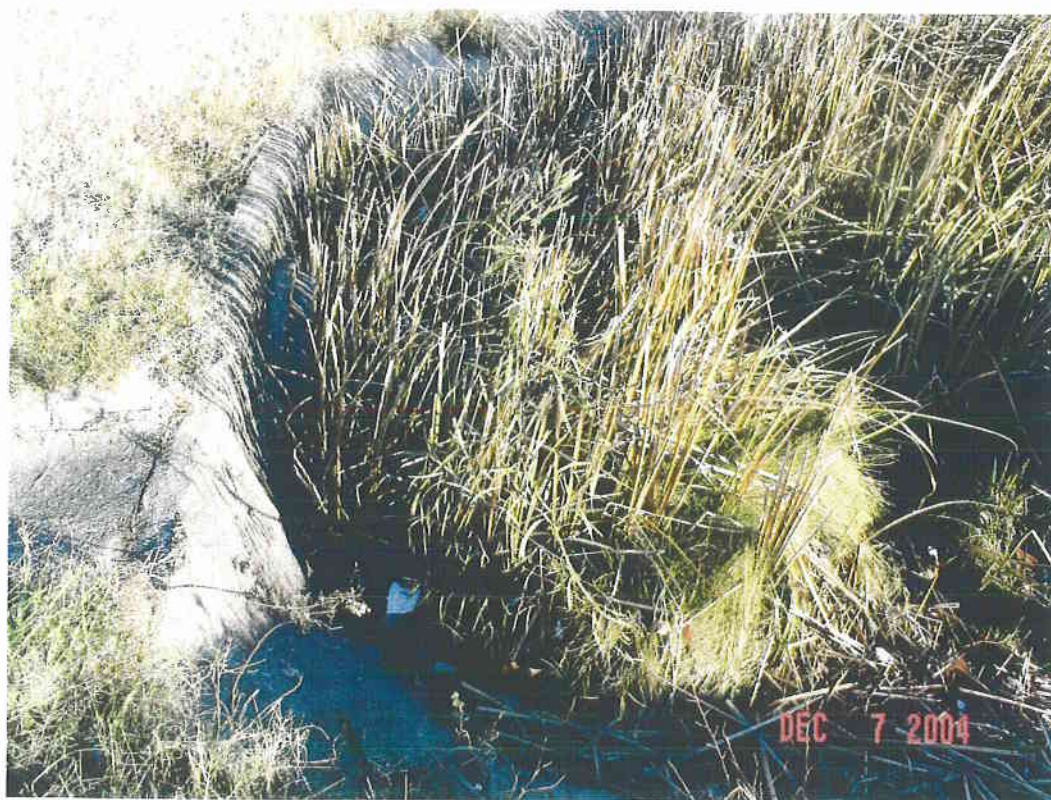
Rancier storm sewer discharge to Long Branch Tributary, blocked by reeds
