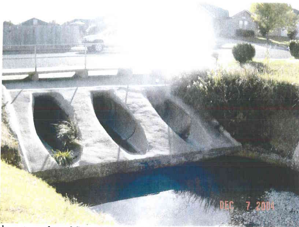
downstream face of Caprock Dr culvert, scour hole
