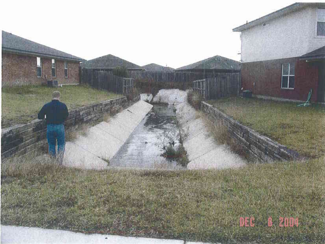
Discharge of storm sewer system into Acorn Creek Morning Star and Acorn Creek Trl
