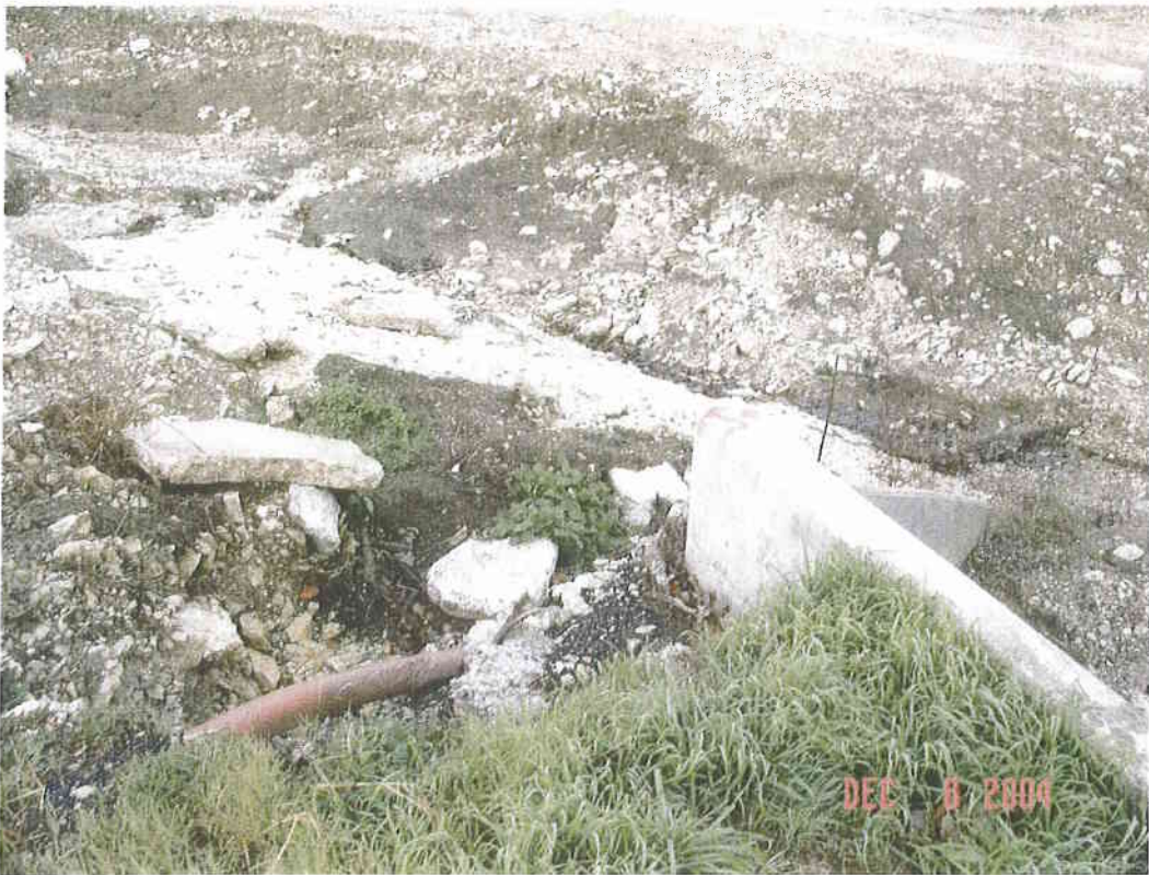
erosion at end of Dripping Springs Dr
