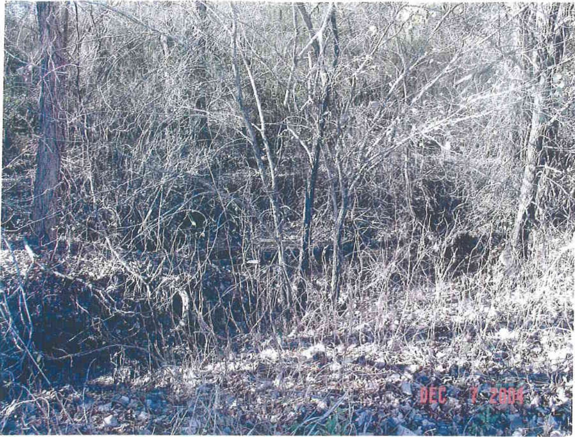
Earthen channel downstream of concrete channel, vegetation overgrown
