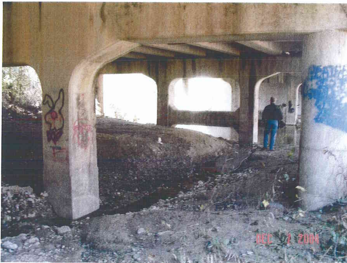
Dogwood channel confluence with LNC under bridge, erosion at piers
