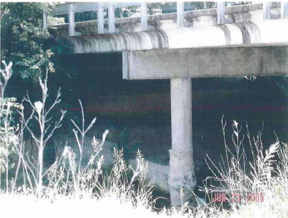
Failed south abutment
