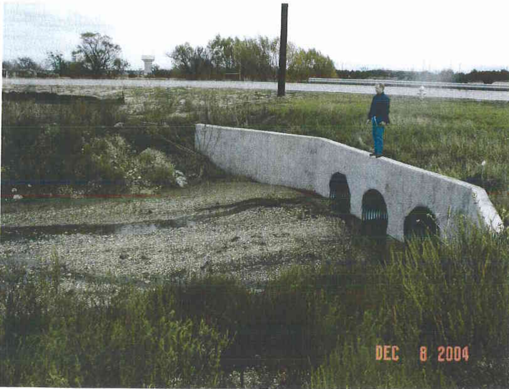
Upstream face of culvert from northwest drainage area WS Young at Schorn Dr
