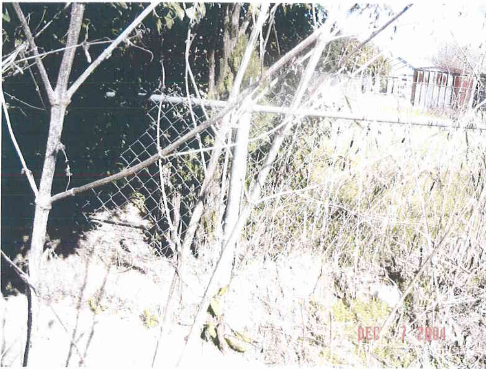
High water mark at end of flume – note debris
