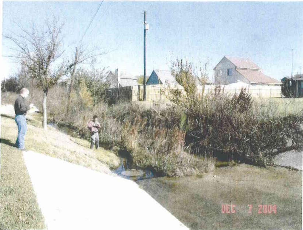
Caprice Ditch upstream of Westcliff Rd, concrete channel being undermined
