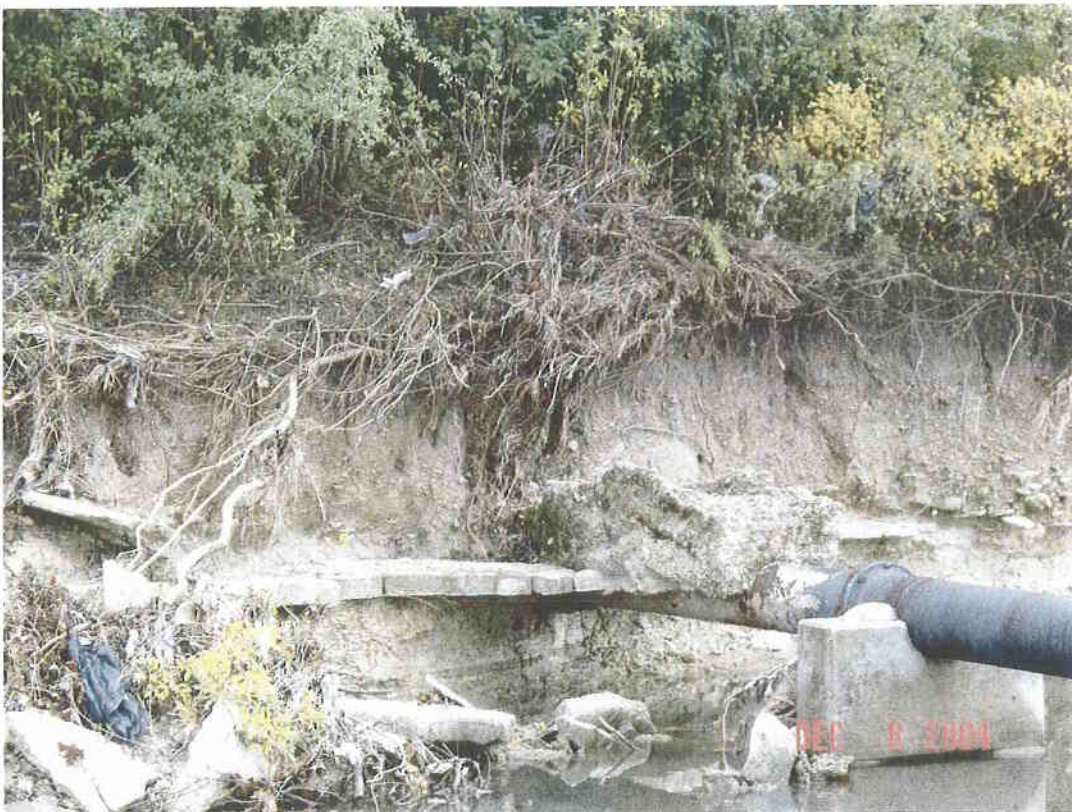
Erosion on right bank near sewer crossing
