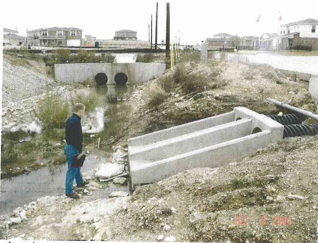
culverts in new subdivision erosion has occurred
