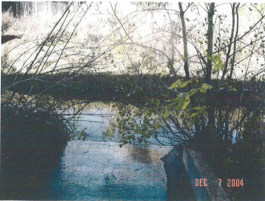
Flume discharging into LNC1
