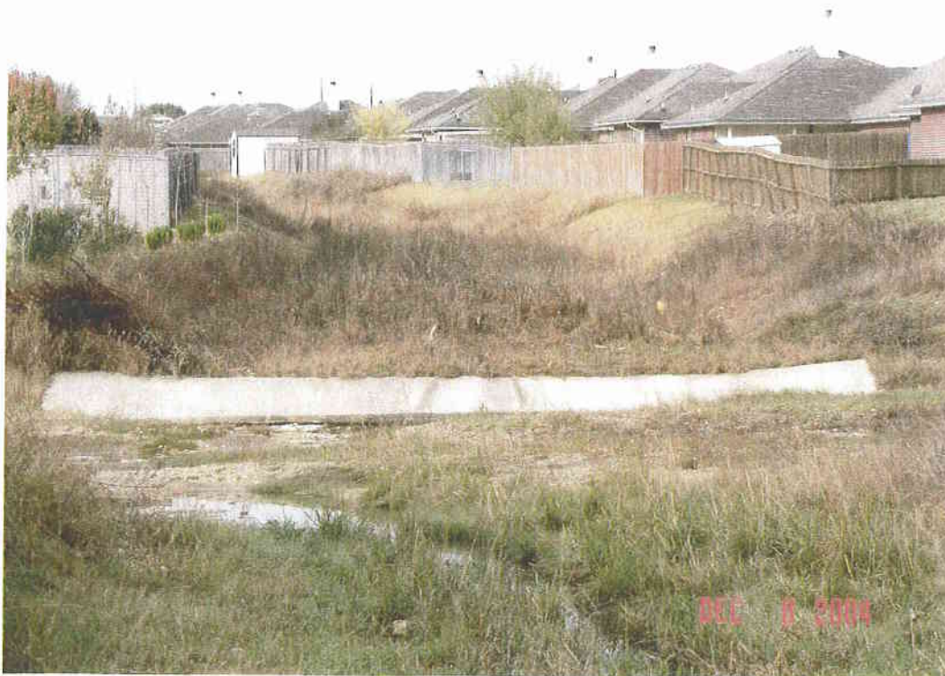
undermined concrete apron for Embers Ditch, West Trib
