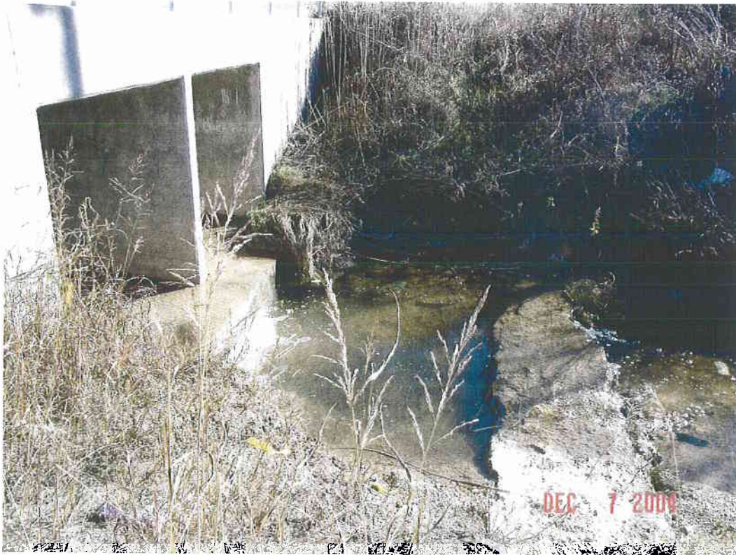
scour at downstream face of Hilliard Ave culvert, concrete encased utility crossing exposed
