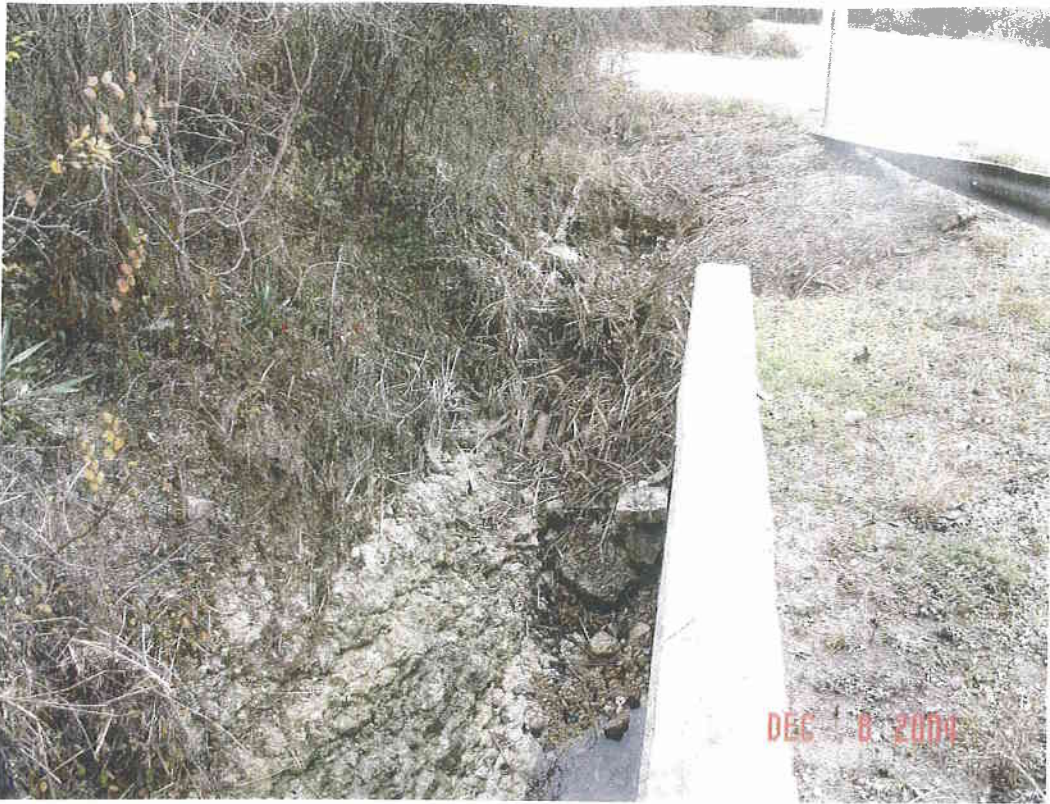
Erosion at northeast headwall
