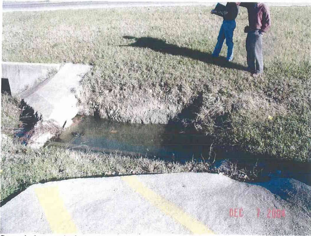
Scour hole at end of concrete flume, just upstream of concrete channel.
