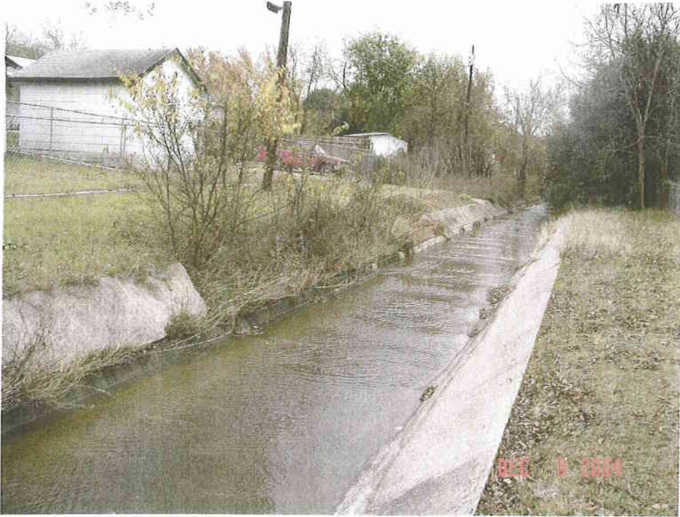
missing concrete section
