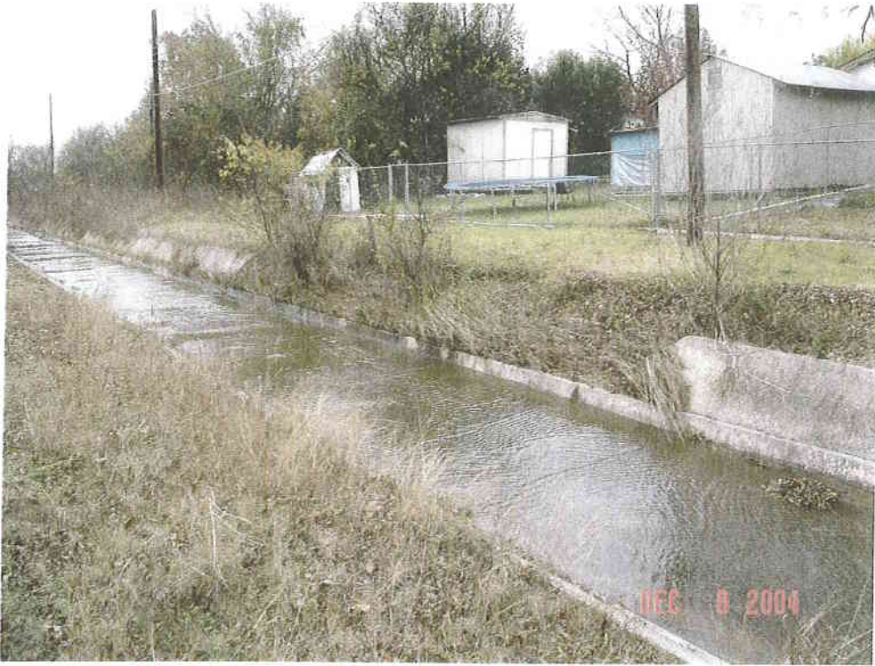
missing concrete section
