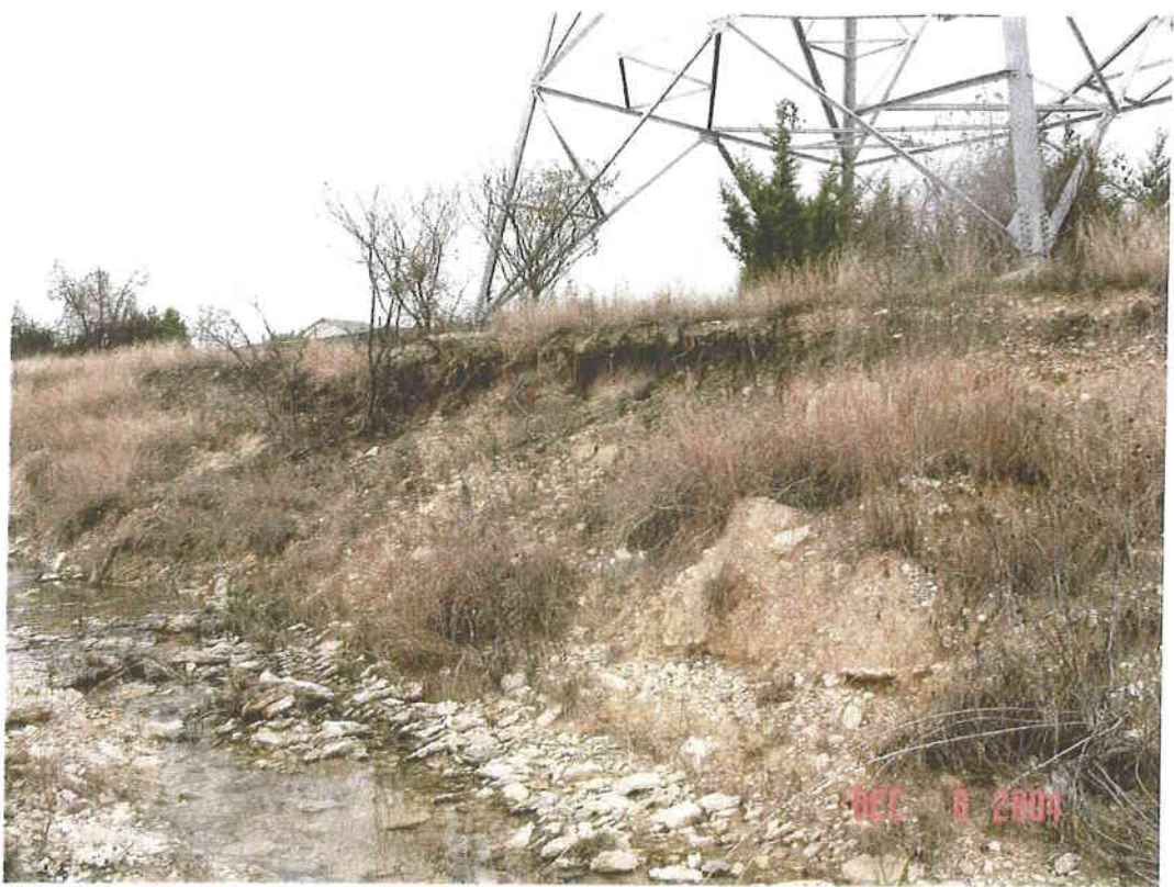
bank erosion at tower
