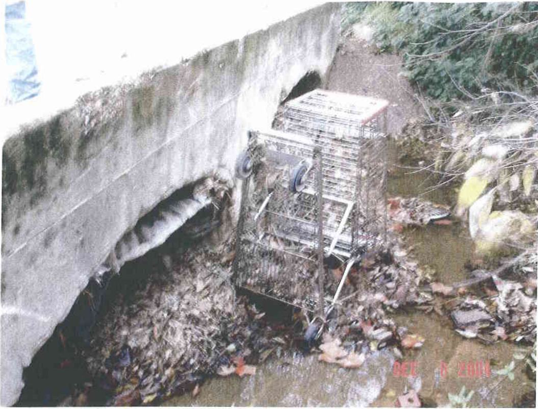
upstream face of Ave C culverts, debris blockage, failure of CMP
