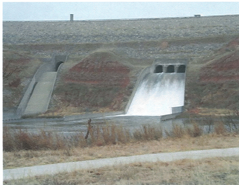
Small Test Release from the Flood Control Outlet Works at Sanford Dam
