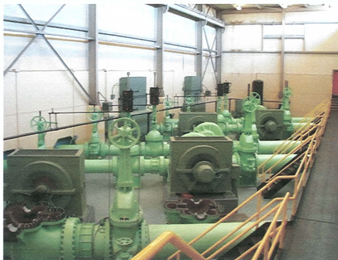
Pumping Plant 1 (5 units @ 1, each)
