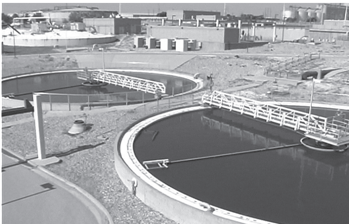
▼ Aeration Basins at the Water Reclamation Plant.
