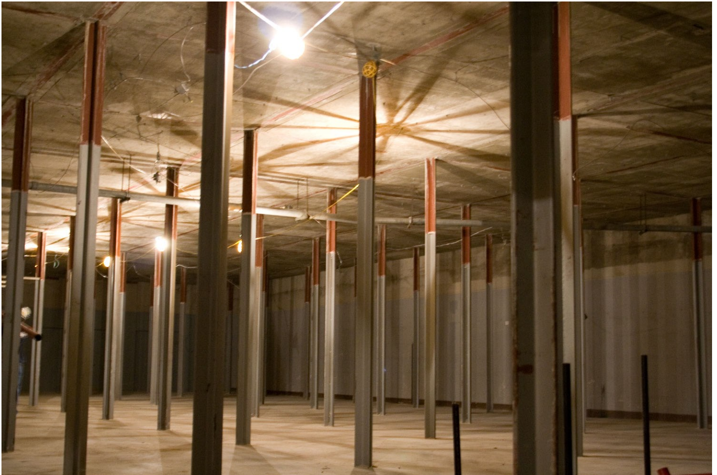
In this photo released by the Texas State Library and Archives Commission, the ground floor stack is stripped of electrical, plumbing and ductwork down to the support beams so that a preaction fire suppression system, new lighting and ductwork, and compact shelving can be installed, July 7, 2008. The TSLAC flagship building is currently undergoing renovation. The 46-year old Lorenzo de Zavala State Archives and Library Building is located at 1201 Brazos Street, Austin, Texas. (TSLAC/Peggy Lee Oster)
