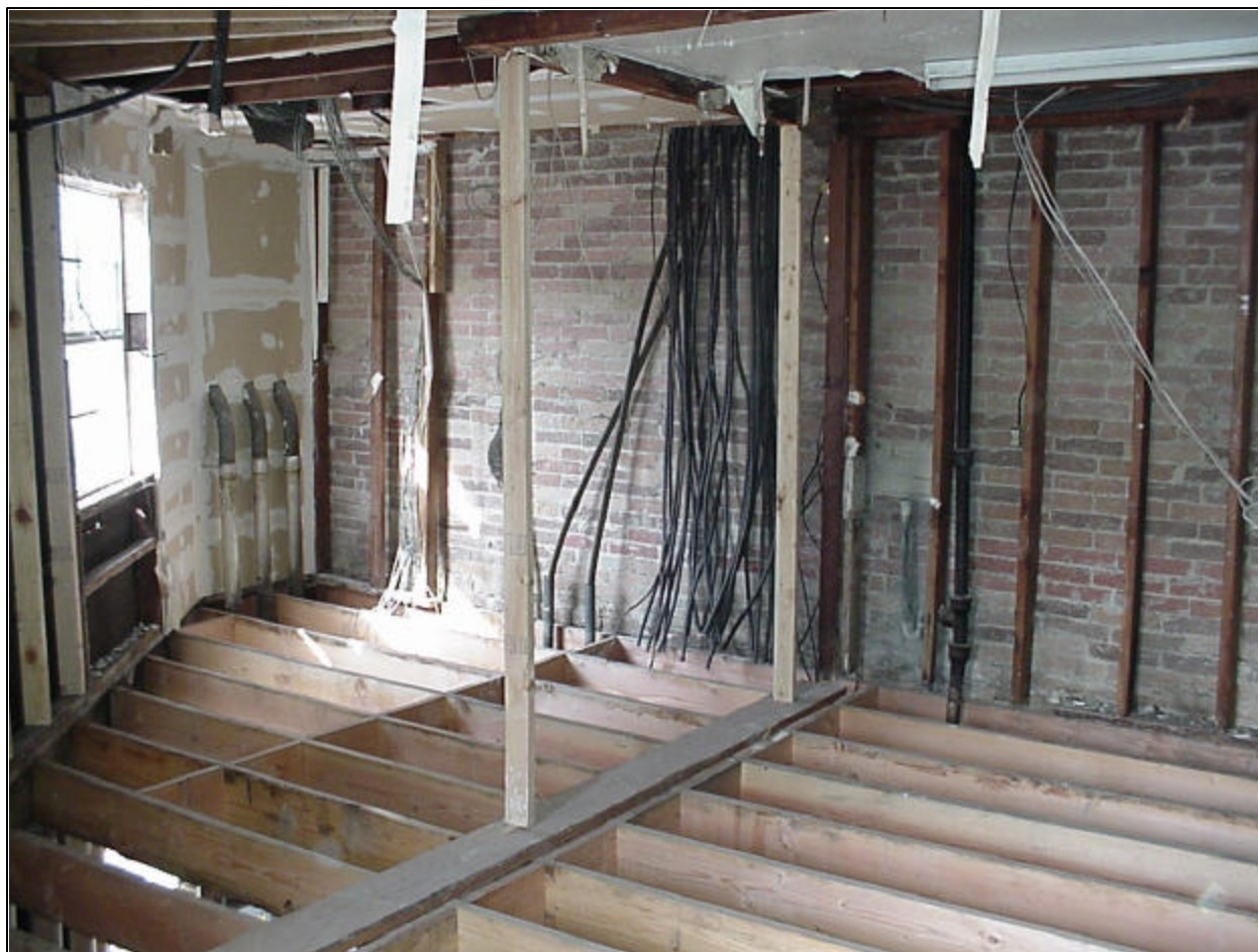
Figure Thirteen. Jacking posts used in second floor of adjacent building undergoing renovation.
