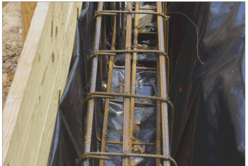
Photo 2. Close up. Vapor barriers create isolation between the concrete and the earth. These are not suitable for use as concrete-encased grounding electrodes.
