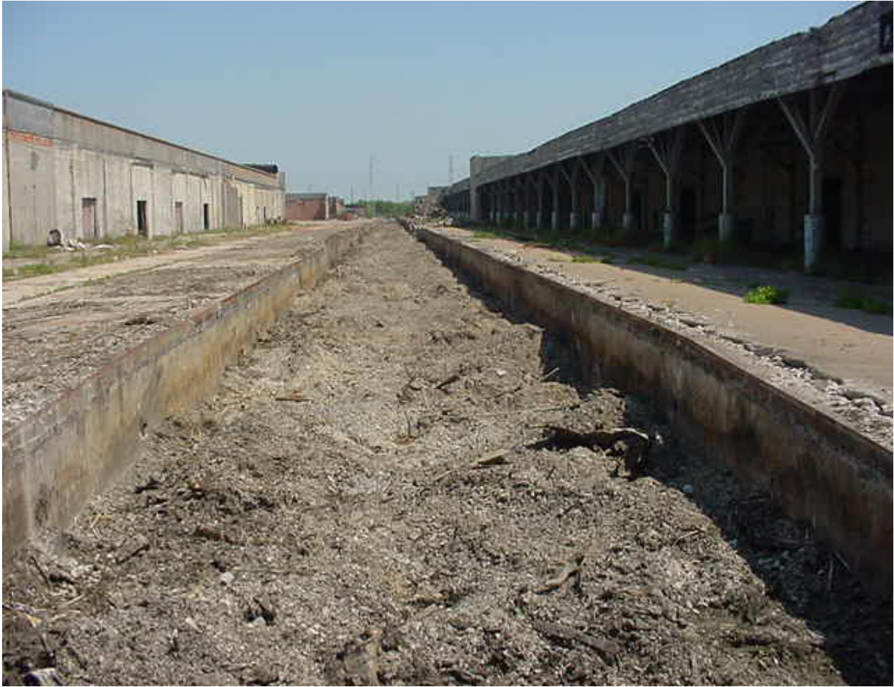
Railroad Tracks Covered with Debris between Loading Docks at the Former Moody Cotton Compress, Site of the Future Galveston County Justice Center 2003
