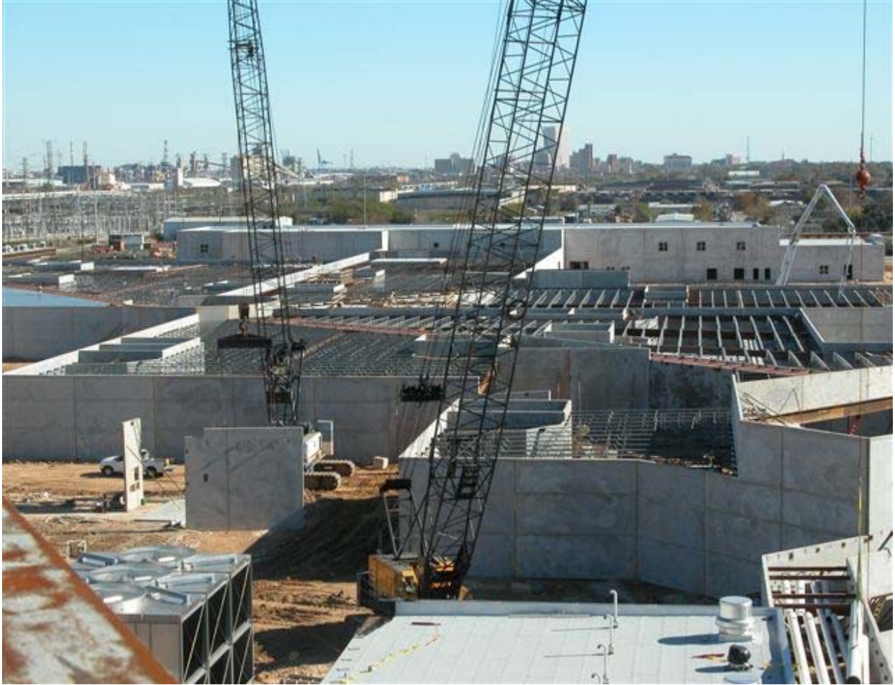
The Galveston County Jail at The New Galveston County Justice Center December 14, 2004
