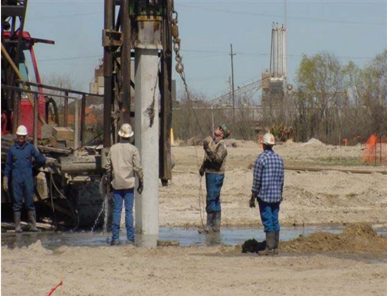
Early Construction at The New Galveston County Justice Center - Workers Drive Pilings on March 8, 2004
