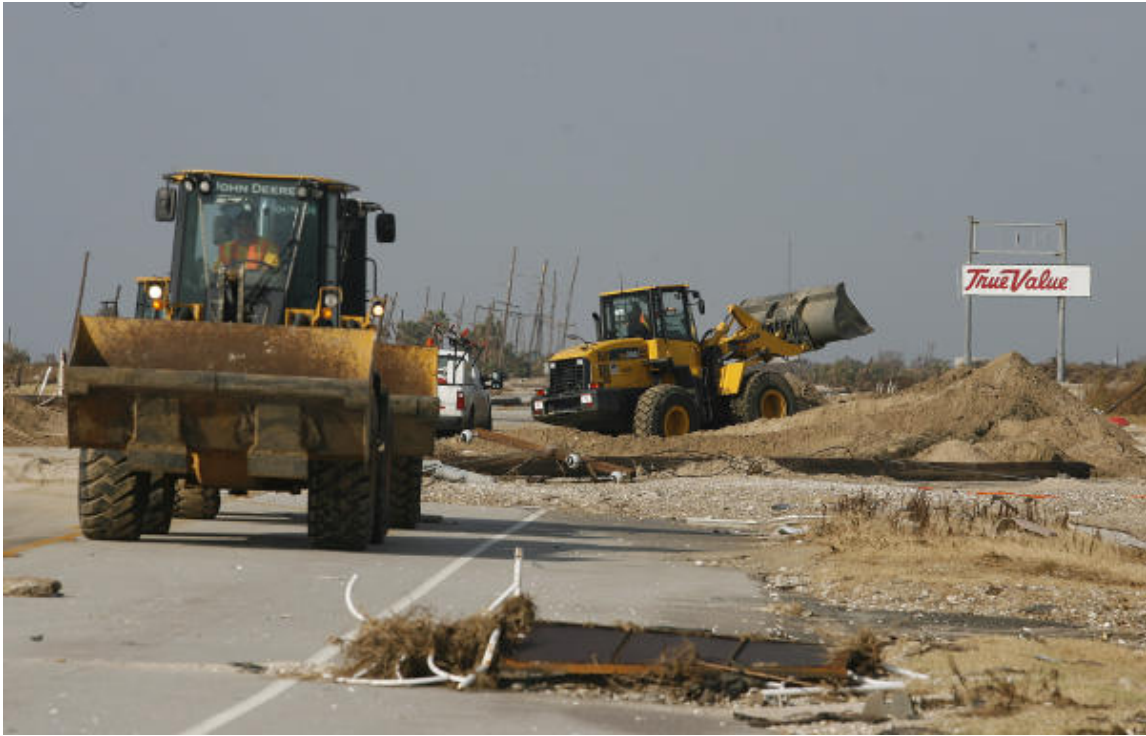
Highway crews cleaning up debris on Bolivar Peninsula.
