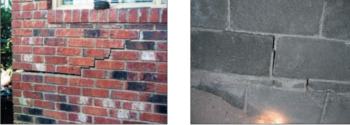
FIGURE 9: MASONRY WALL CRACKS
