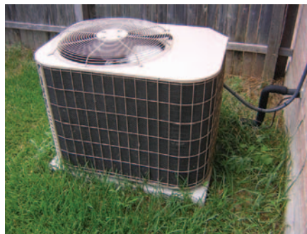
FIGURE 20: OUTDOOR PORTION OF AIR CONDITIONING UNIT
