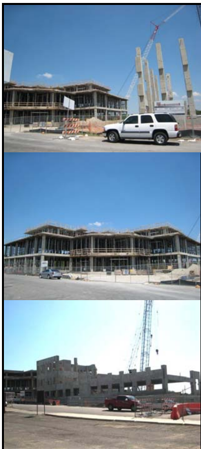
Construction on the new justice center and parking garage is progressing and hopefully all will be complete by April, 2010.
