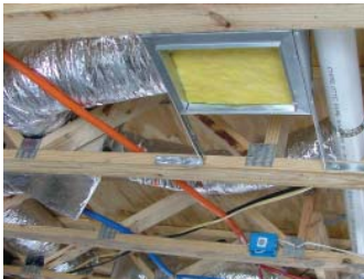
There are six Building and Mechanical programs under TDLR, including Air Conditioning and Refrigeration Contractors
