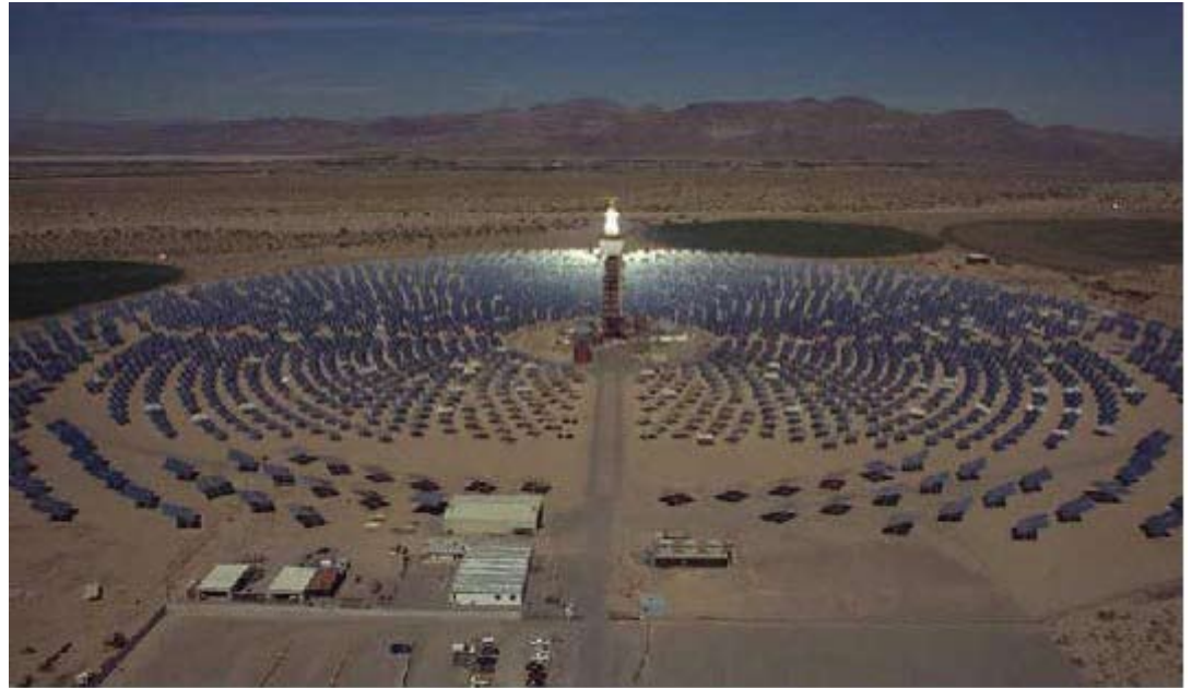
EXHIBIT 3-14 Solar Two (central receiver design)
